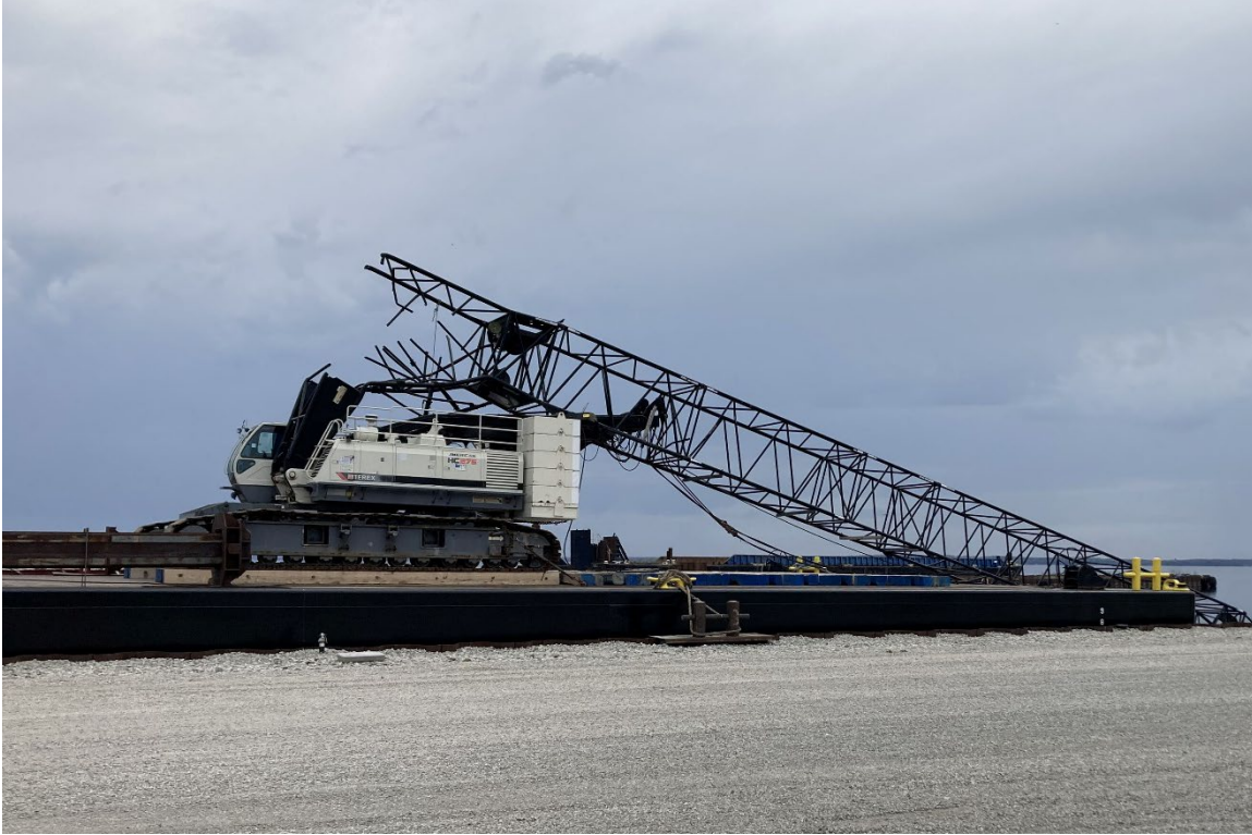
Figure 7. The boom bent backwards over the cabin after striking the bridge. (Source: Coast Guard)
