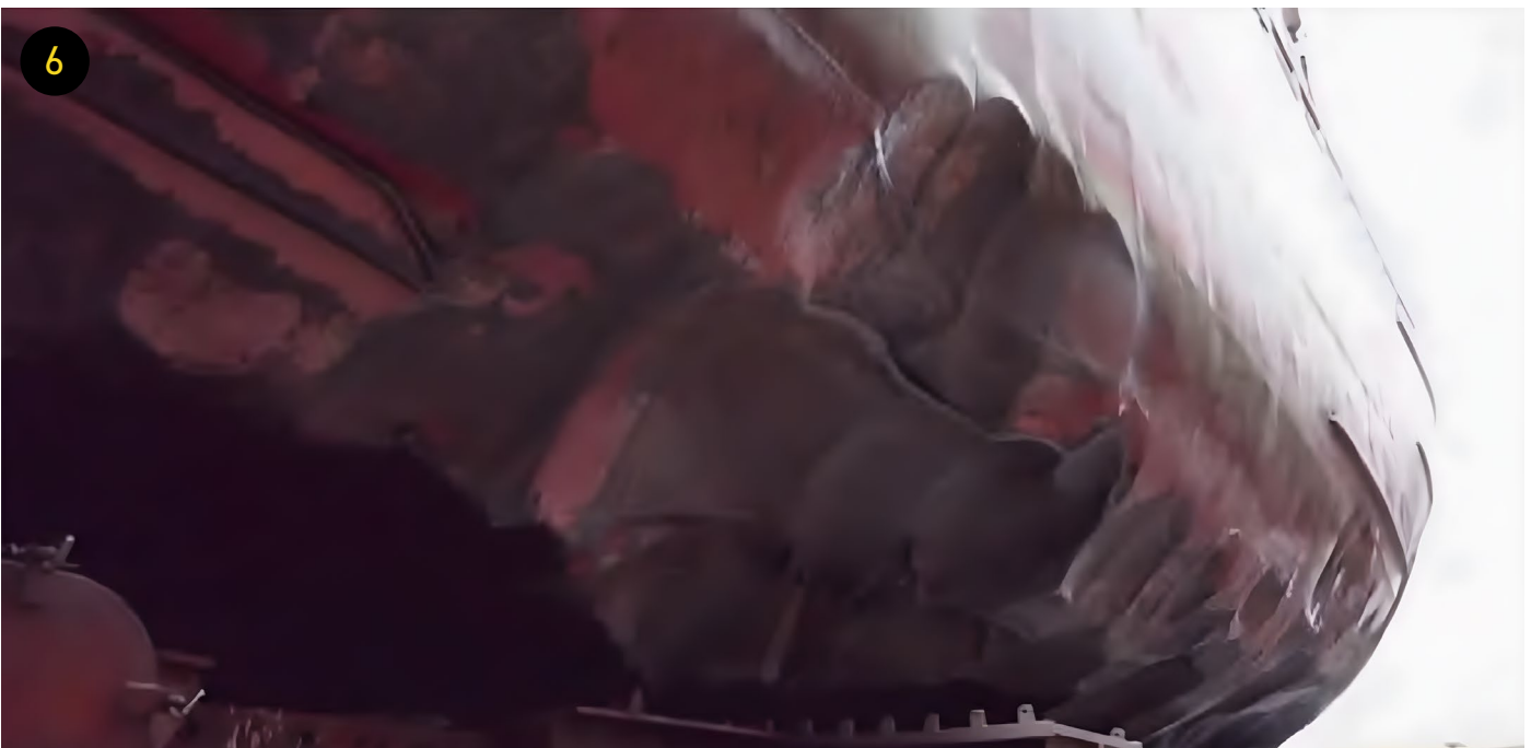
FIGURE 6 SIGNIFICANT DAMAGE AROUND THE MIDSHIP STARBOARD SIDE SOURCE REPUBLIC OF BULGARIA NAMRAIB
