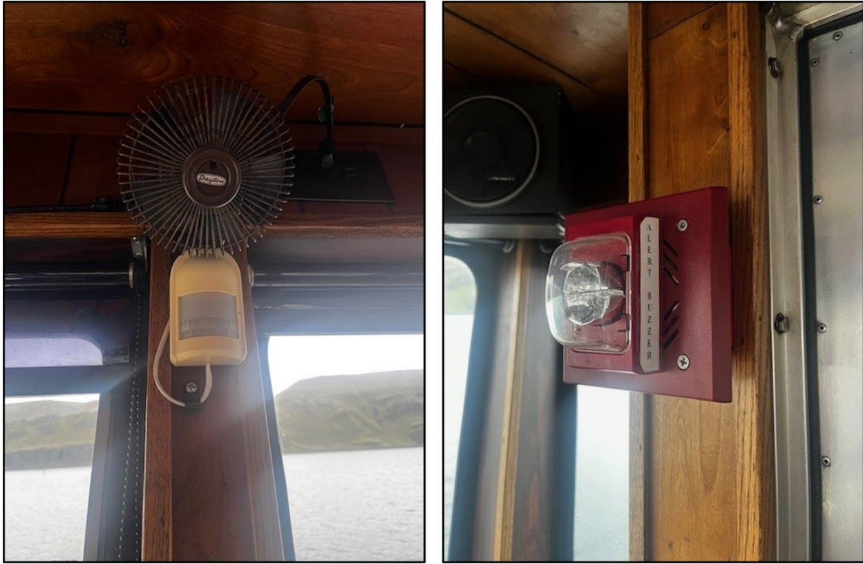
Figure 7. Left to right: Cindy B pilothouse alerter system motion detector (one of two on board) and strobe light with audible alarm. (Source: WCP Inc.)
