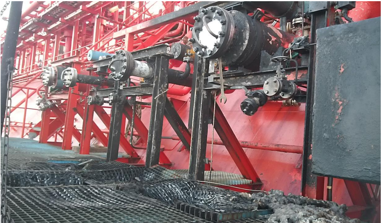
Manifold with steel spanner attached post-fire
