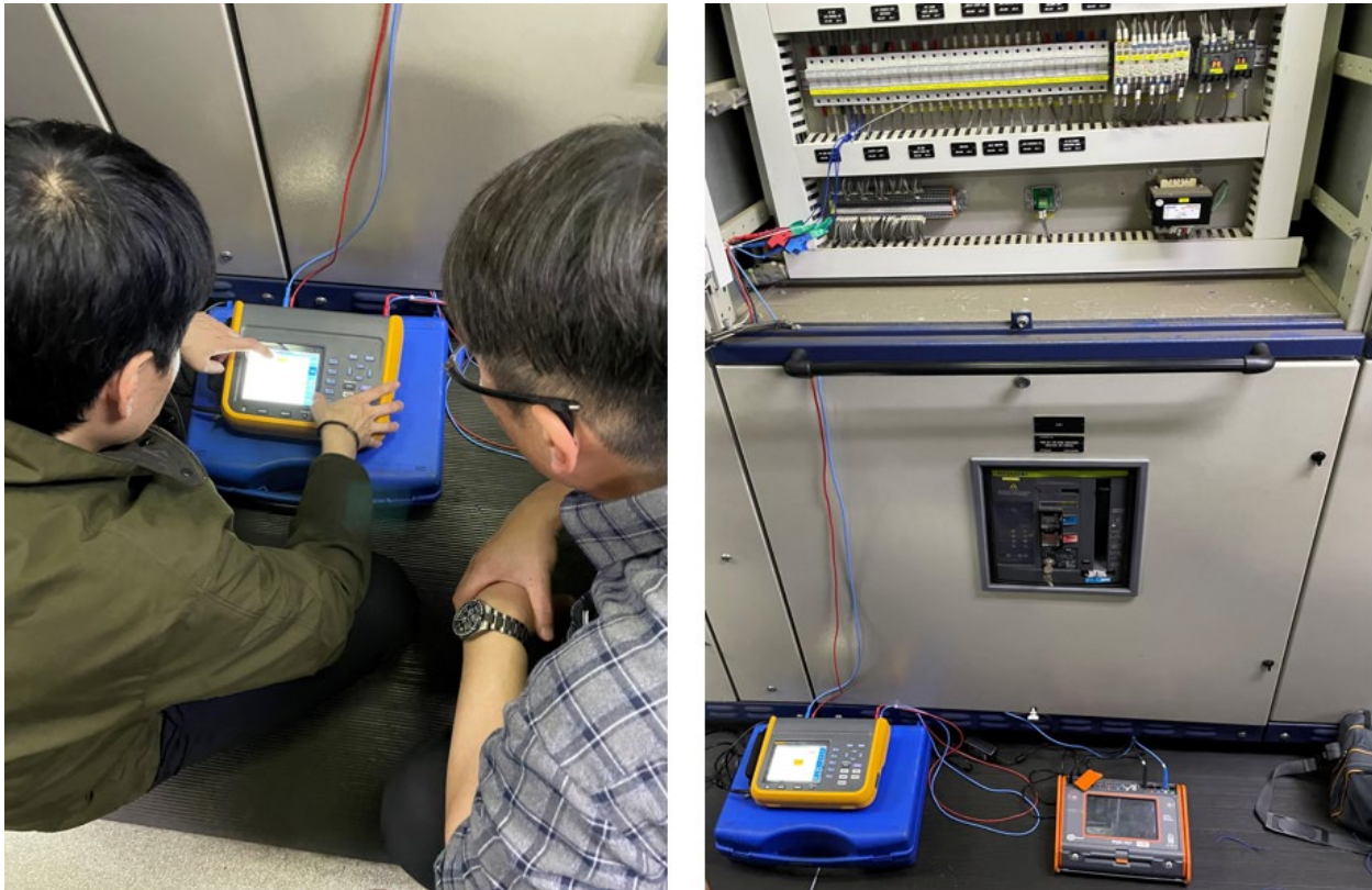
Figure 3. Left to right: HHI electrical engineers installing and monitoring the power analyzer connected to the LV switchboard. The power analyzer fully connected to and monitoring the LV switchboard.
