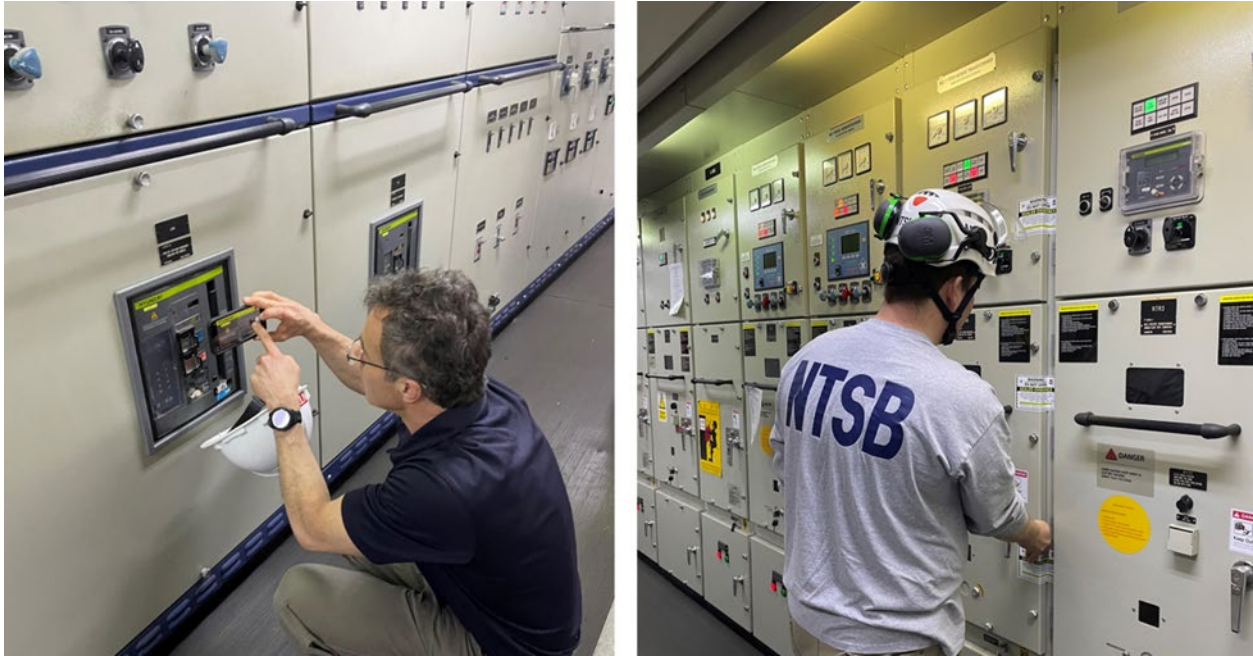
Figure 1. Left to right: An NTSB investigator examines a circuit breaker on Dali 's low-voltage (LV) switchboard, and an NTSB Investigator applies tamper-evident preservation seals to the HV switchboard.
