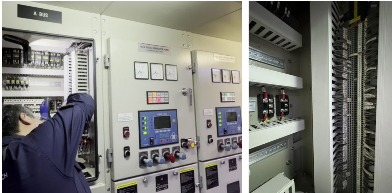
Figure 4. Left to right: An HHI engineer inspects wire connections within the HV switchboard. Also shown, terminal block arrangement with individual wire connections.
