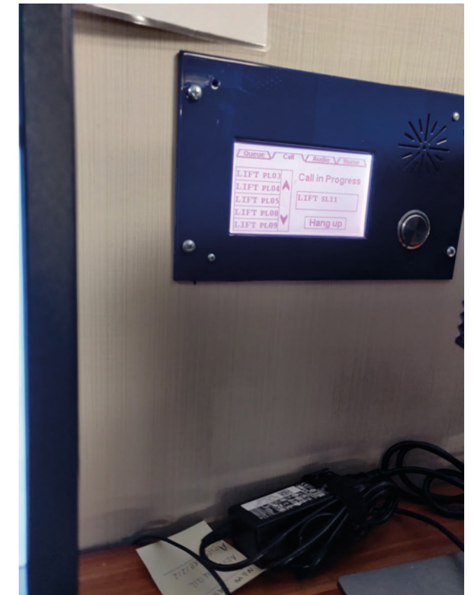
FIGURE 40. Passenger elevator alarm panel hidden behind a desktop screen in the ECR
