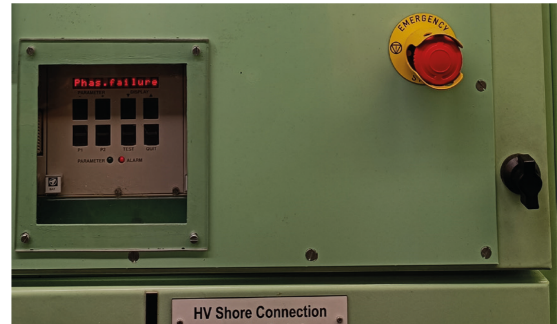
FIGURE 33. Phase failure alarm for the HV shore connection panel – while underway, disconnected and many miles from shore
