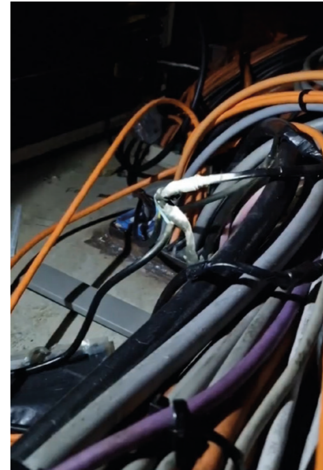
FIGURE 52. The T-connection or “power thief” upstream of the UPS supplying the navigational systems
