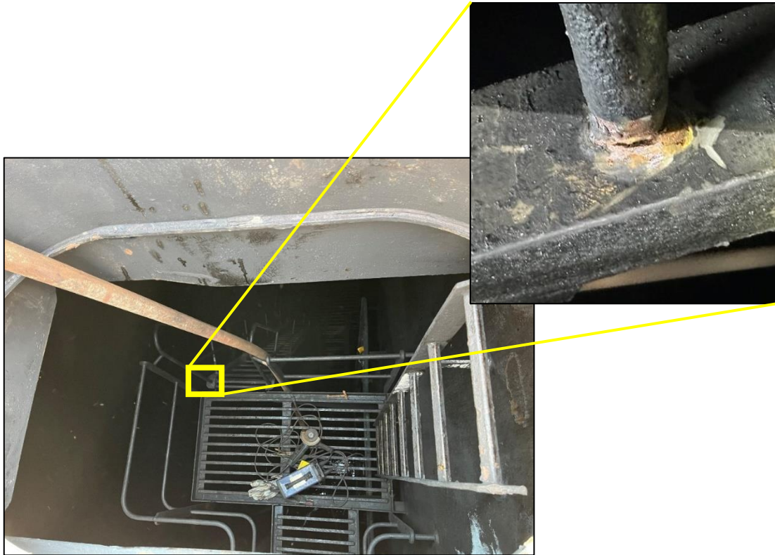
Figure 8: entrance to port side lope tank, showing the first stanchion that required repairs
