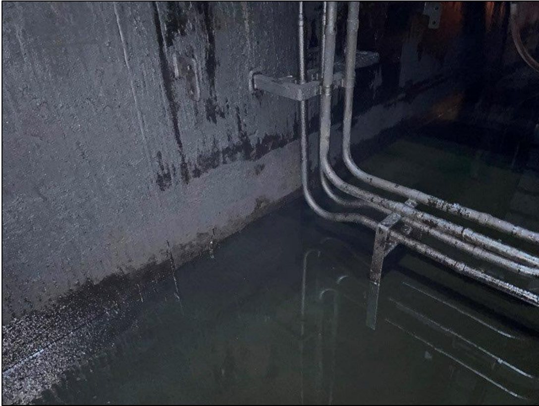
Figure 13: Firefighting water inside the slop tank
