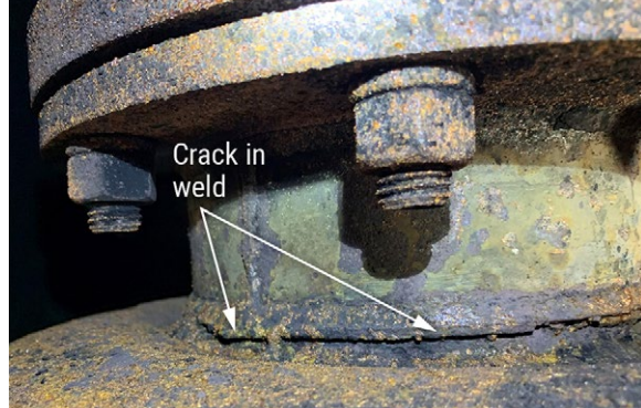
Crack in weld below the upper (outlet) flange of the starboard muffler aboard the Mary Dupre . SOURCE: NTSB
