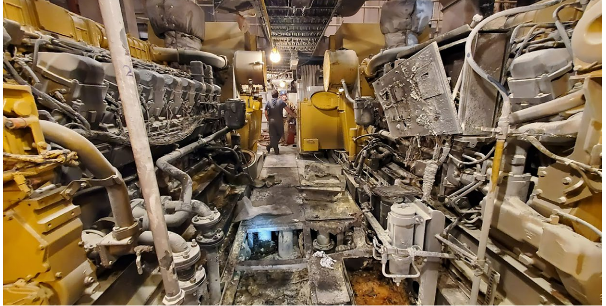
The walkway between the nos. 3 and 4 main engines after the engine failure and fire (looking forward). SOURCE: NTSB
