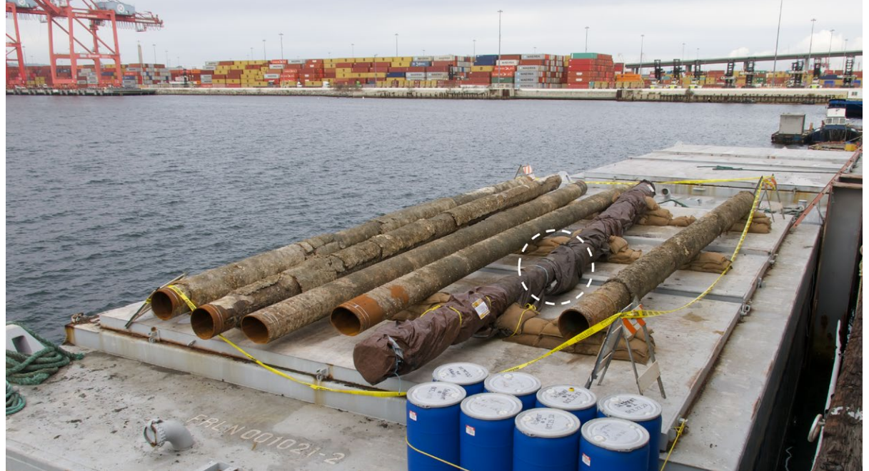
Six segments of damaged pipeline removed for replacement. The leak site (circled) was observed on the segment shown wrapped in a tarp. SOURCE: NTSB
