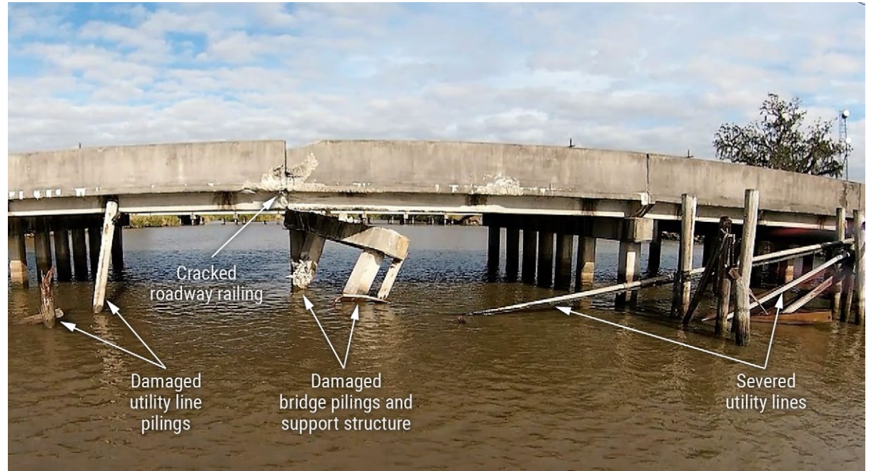
Route 182 bridge damage. BACKGROUND SOURCE: CAJUN DRONE PHOTOGRAPHY, JIM PIERCE JR.
