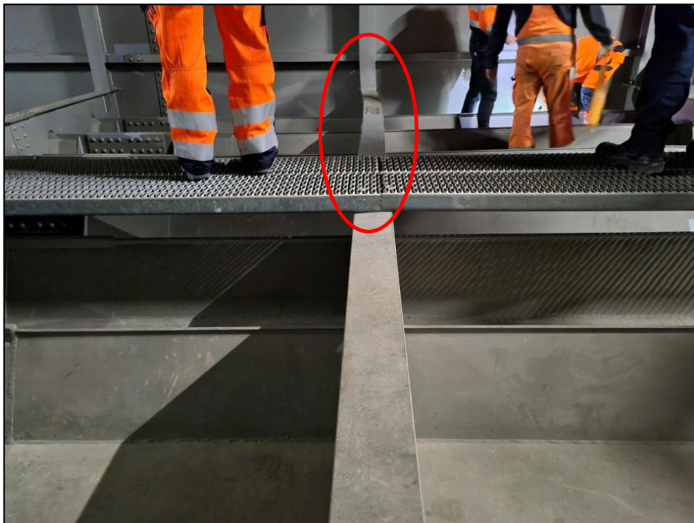
Figure 20: Deformed hollow box girder (Olympiabrücke bridge) 28
