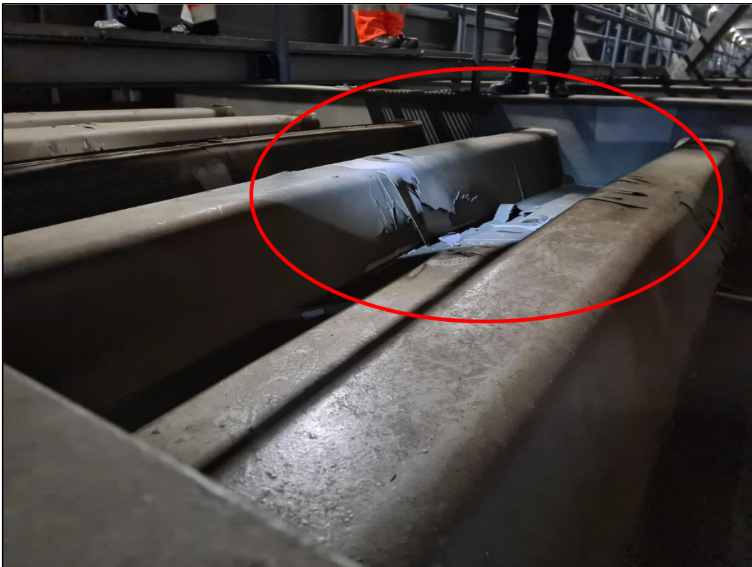
Figure 22: Damaged hollow box girder (Prinz-Heinrich-Brücke bridge) 30
