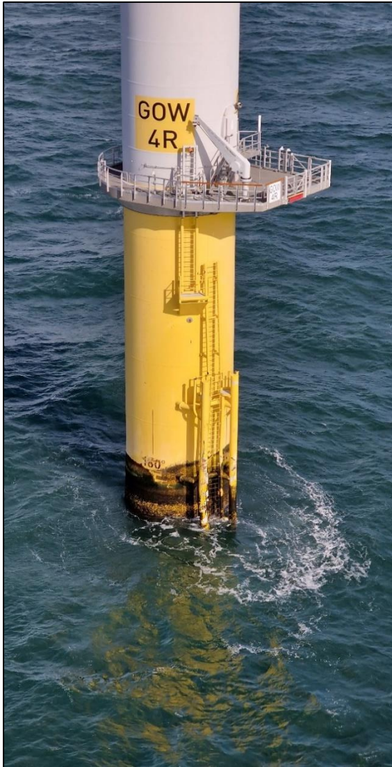
Figure 8: Base of the wind turbine with which the allision occurred 14
