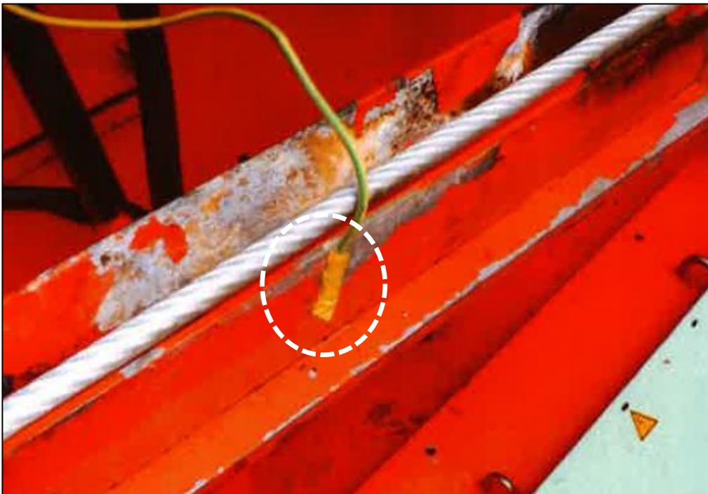
Figure 24: Female tab connector (wrapped in insulating tape) detached from the male tab connector on the inside of the cover
