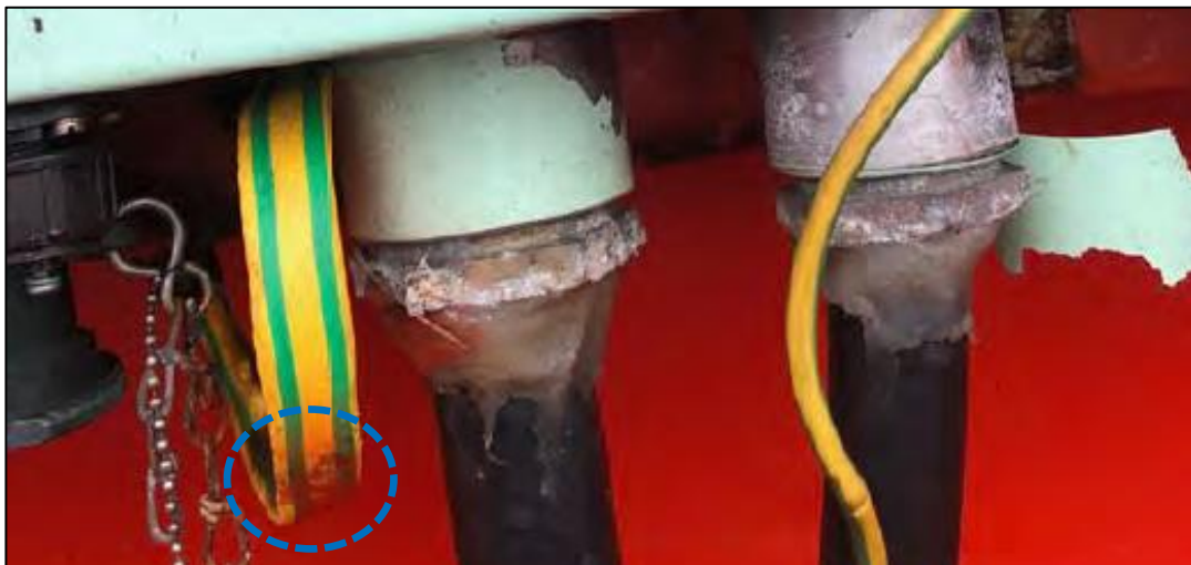
Figure 14: Corroded section of the main earth lead below the housing box 17
