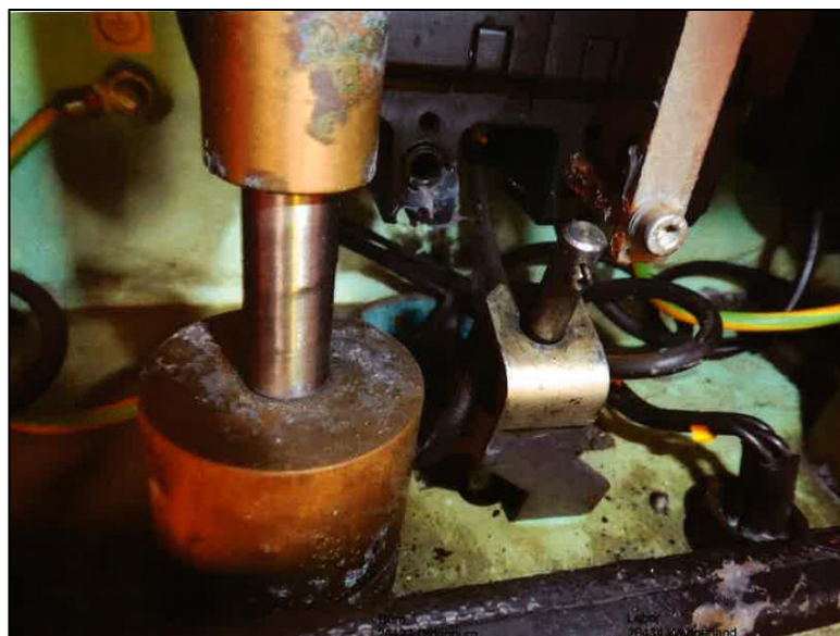
Figure 19: Traces of corrosion on the switching rod inside the switch box
