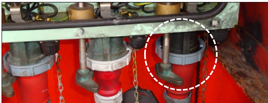
Figure 22: Socket base in the terminal/switch box at bay 38/39
