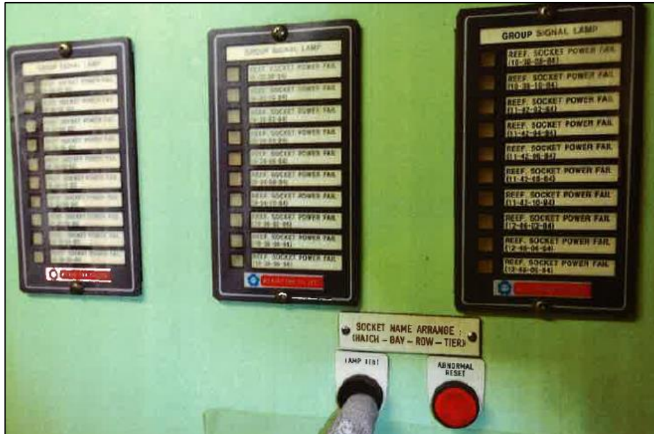
Figure 18: Panel on the power supply cabinet
