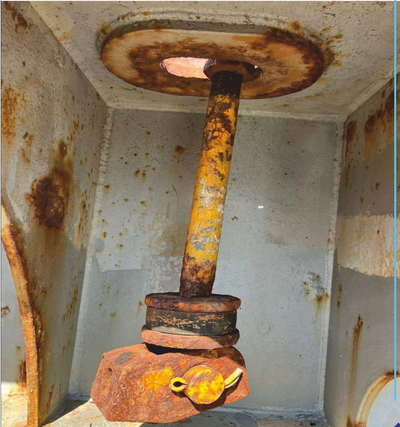
Hatch covers hydraulic pipes heavily corroded
