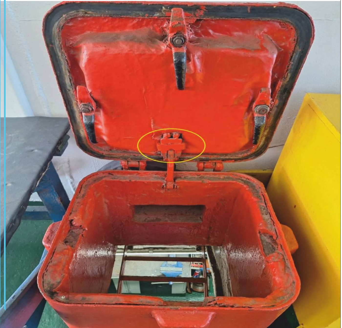
Safety Lock of Engine Room Emergency Exit Door is Seized
