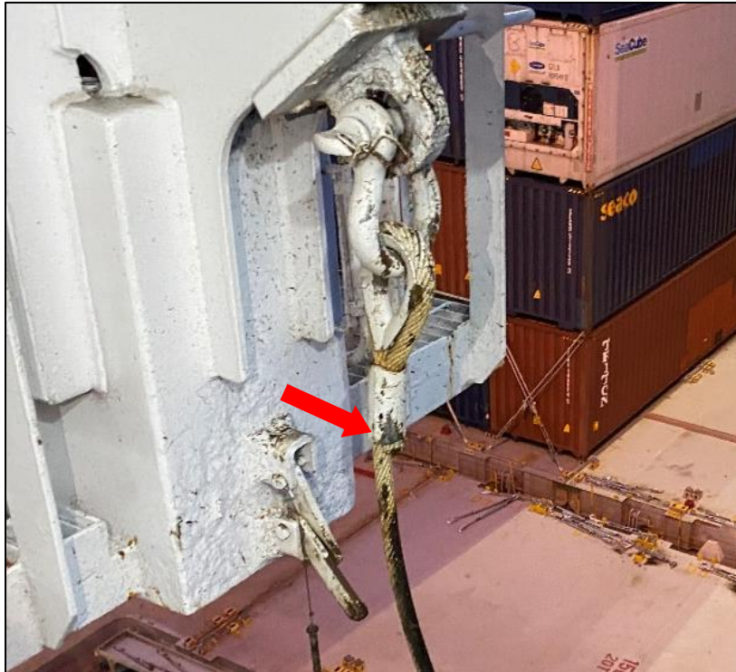
Figure 10: The abrasion marks (red arrow) observed on the ferrule at the fixed end of the parted wire rope
