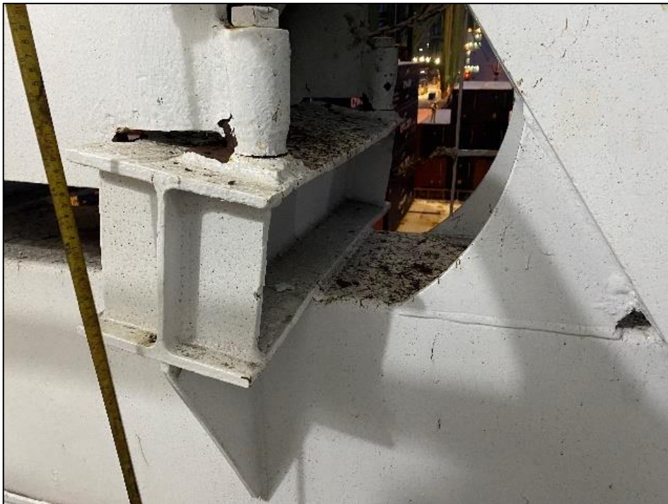
Figure 7: The damaged port side winch foundation
