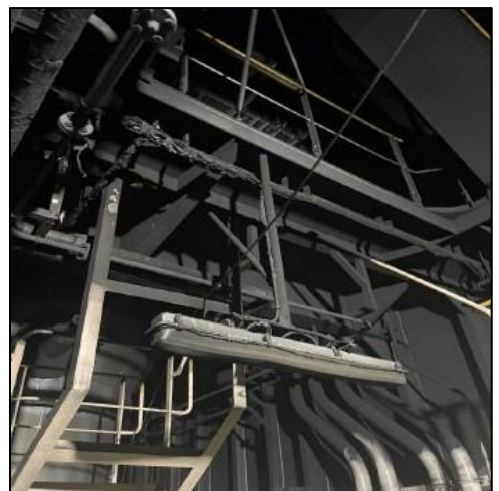
Figure 10: Burnt power cables and a lighting fixture outside the transformer room
