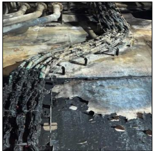
Figure 9: Burnt power cables outside the MVSB room
