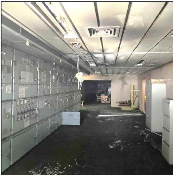
Figure 7: The MVSB room
