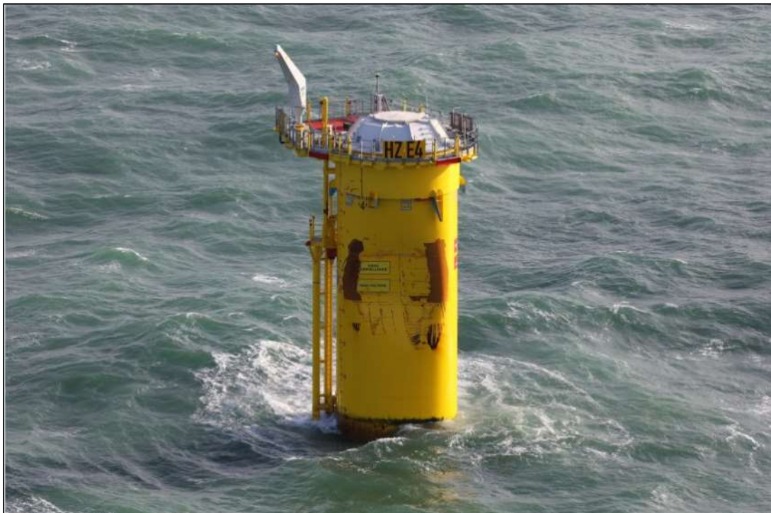
Figure 32: Aerial photograph showing some of the damages to the transition section of windfarm foundation HZ E4
