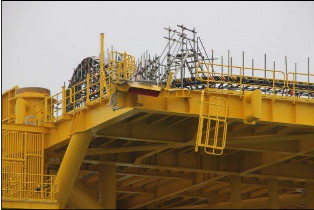
Figure 33: Part of the damages to HZB
