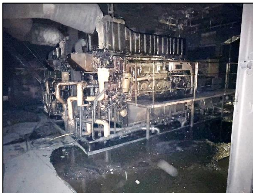
Figure 11: Auxiliary engine (starboard side)
