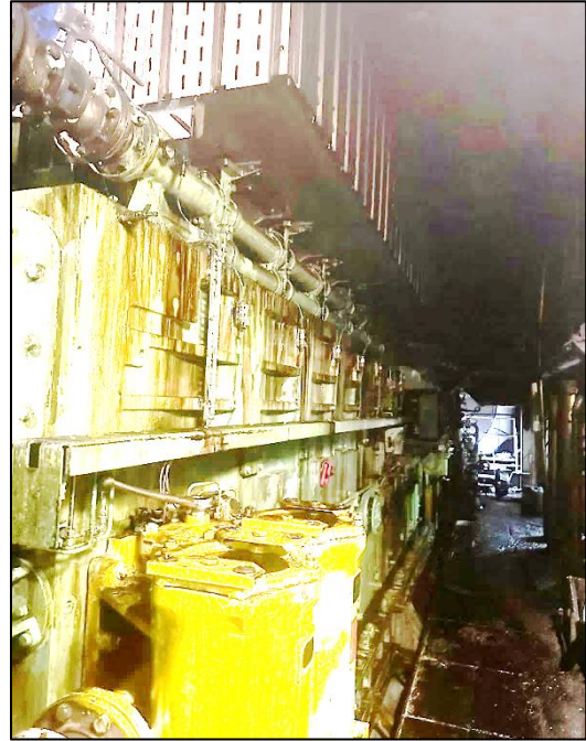
Figure 10: Main engine view forward
