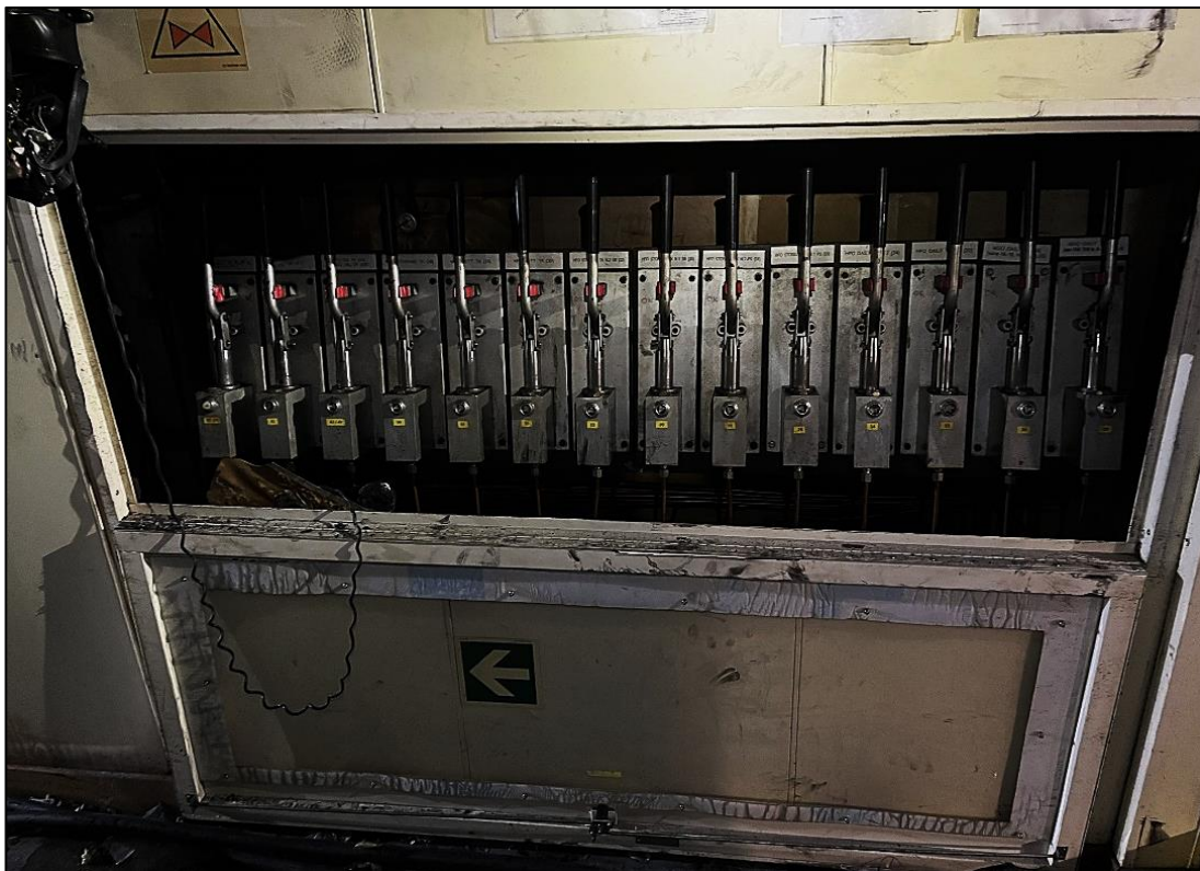
Figure 7: QCV cabinet located outside the ECR
