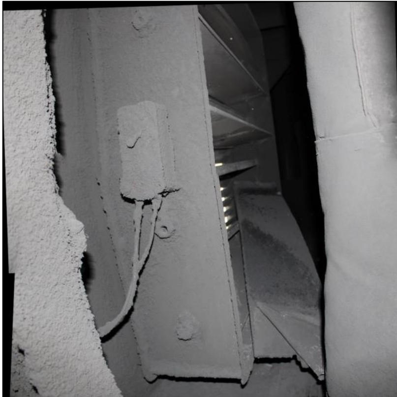
Figure 18: Lowest louver covered in soot
