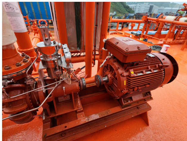
Figure 2.11 – Discharge Booster Pump
