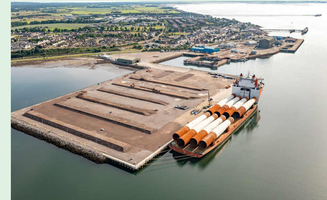
Monopiles arrive for marshalling at Invergordon in the Cromarty Firth, Scotland, during the summer of 2023. These have been deployed onto the 882 MW Moray West project expected to deliver first power in May 2024. In a period of turbulent times for the UK wind industry, Moray West is the only Allocation Round 4 project to have reached financial close through non-recourse project financing, securing GBP 2 billion pounds, and is the first wind farm in the UK to have most of its offtake secured through corporate power purchase agreements. Photo: © Ocean Winds
