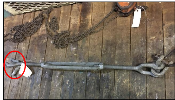
Figure 7: Photograph of the turnbuckle with the securing pin out of place at one end (red circle)
