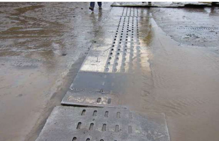
Overflowing primary drain line
