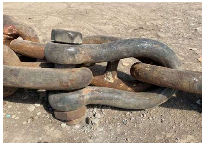
Example of deformed pin and connecting plates in the pulling system arrangement
