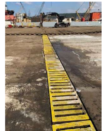
Drainage line, and drainage sump area Source: Site Inspection Report of Dörtel (19.9.2022)
