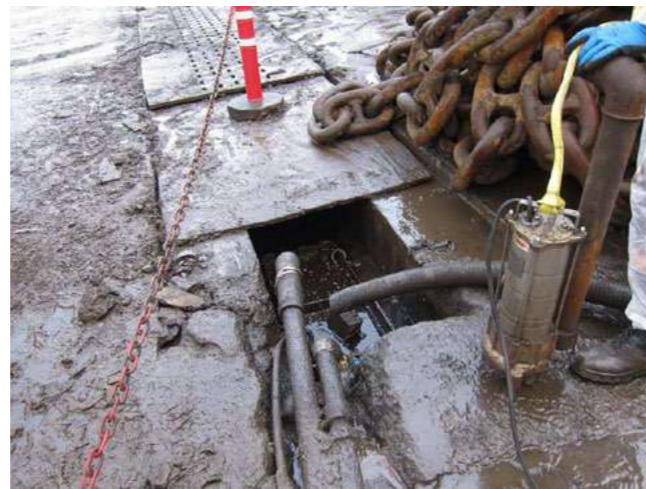
Drainage system pump was out of function
