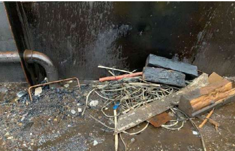
Debris onboard the vessel being dismantled Signs of fires were present Source: Site Inspection Report of Dörtel (5.6.2023)
