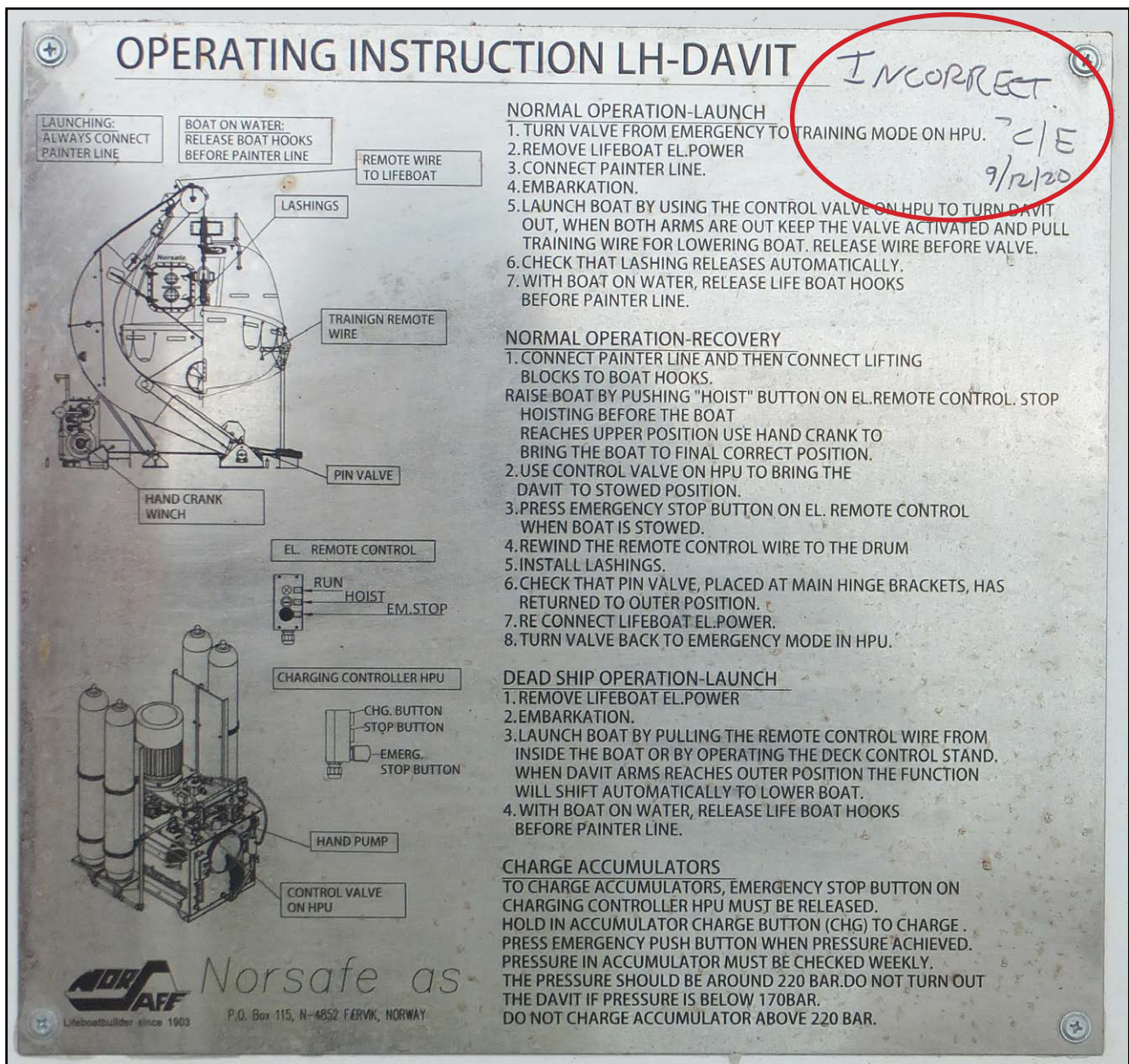
Figure 11: Instruction plates fitted adjacent to lifeboat davits, showing the handwritten statement
