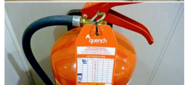
Fire-fighting equipment maintained, routinely inspected and ready for immediate use.
