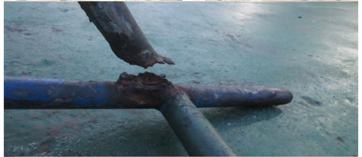
! Both ladders are damaged. The first one is missing the top three rungs and is unsecured.
