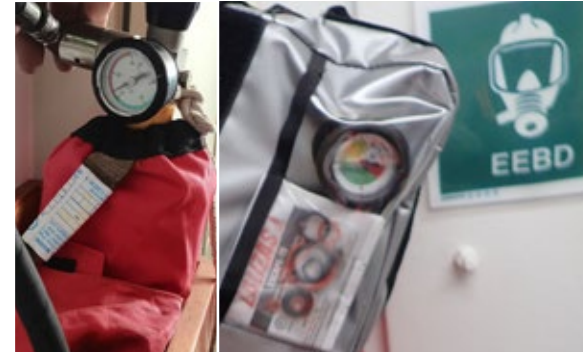
! EEBD gauge indicating an empty cylinder.
