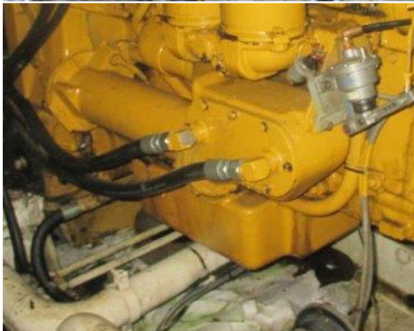
! Oil leaks, including small ones, should be rectified as soon as possible. Oil-soaked absorbent pads increase fire risk
