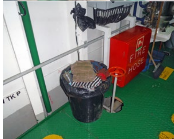
! Machinery spaces should be clear of combustible materials and waste. Garbage receptacles should be metal with a lid. Oily rags should only be placed in metal bins with a lid.
