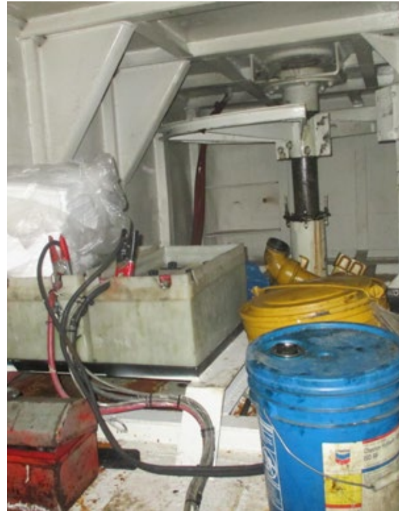
! Exposed batteries along with combustibles, chemicals and other disorganised equipment in steering gear compartment.
