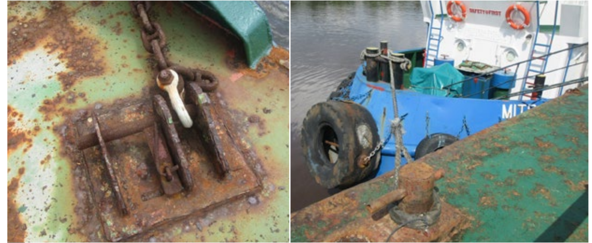
! Deck fittings should be maintained and steel coated to prevent wastage.
