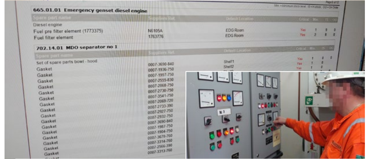
! PMS maintenance routines and inventory and testing of stand-by equipment.
