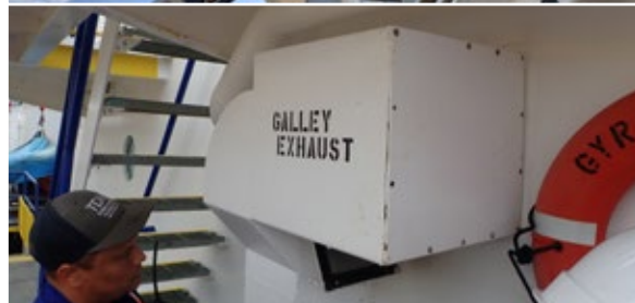
Fire flaps and dampers maintained in good operable condition, clearly signed and labelled.
