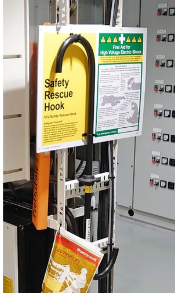
! Rescue equipment and first aid instructions posted in locations where there is a risk of electrocution
