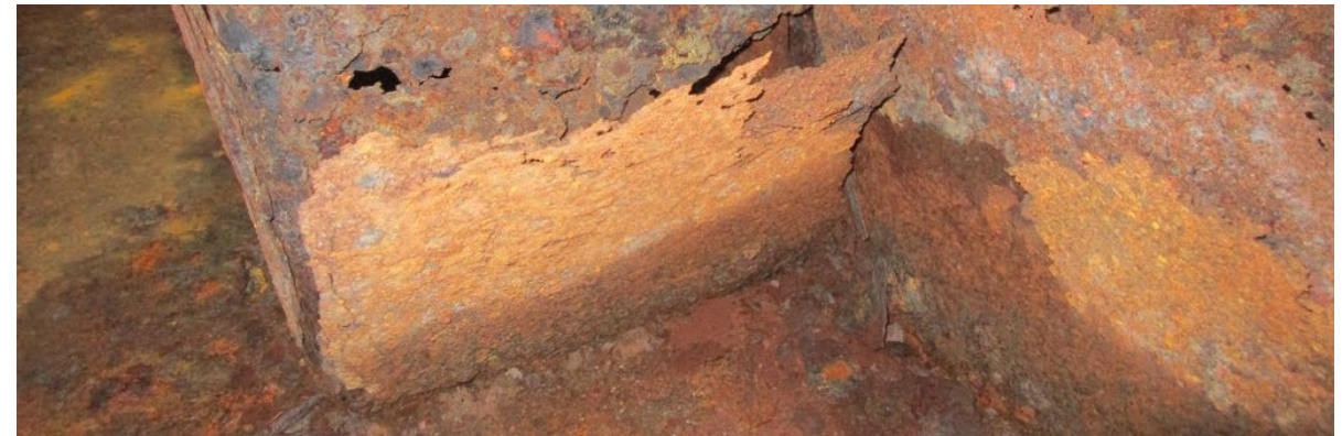
! Well-maintained equipment may look to be in good condition but can be ripped off the deck if the deck and underside structures are allowed to waste.
