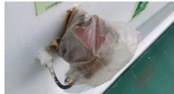
! Emergency stop not weather-tight.
