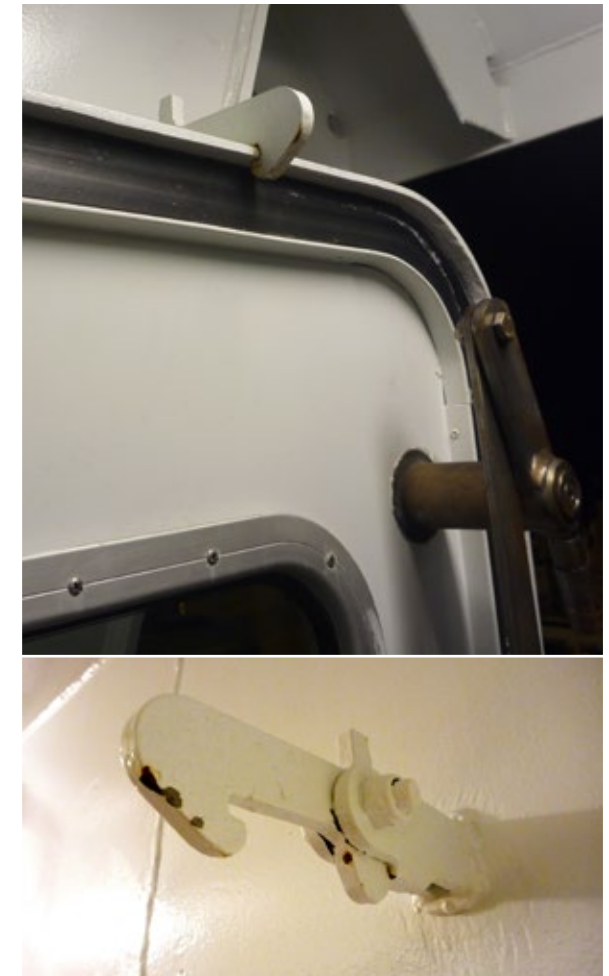
! Hold-back devices installed so that doors can be safely secured in the open position.
