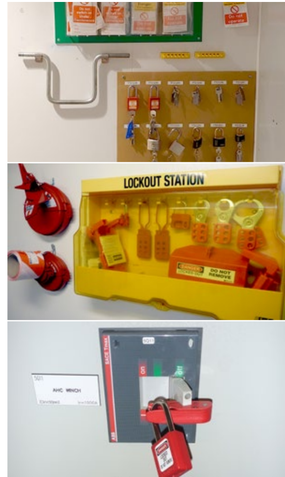
! Lock-out tag-out (LOTO) equipment available for system isolations, including a range of valve and switch locks.
