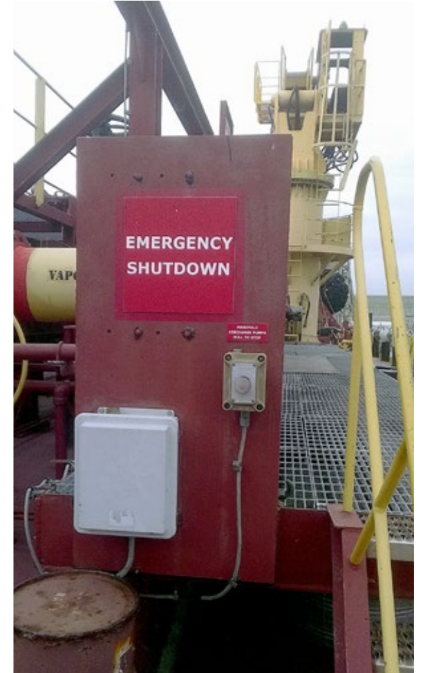
! Emergency shutdown and emergency stop buttons clearly signed.
