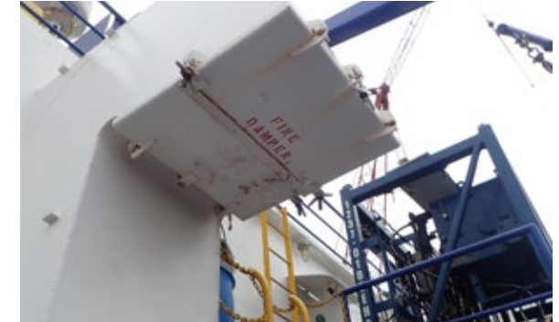
! Vent flap not marked to indicate the space/compartment served.
