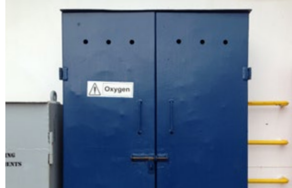
! Gas cutting/welding cylinders (Ac/Ox) and any domestic fuel gas cylinders stored securely in a protected and ventilated space outside of the accommodation. For gas distribution systems, safety devices in use as per certified installation
