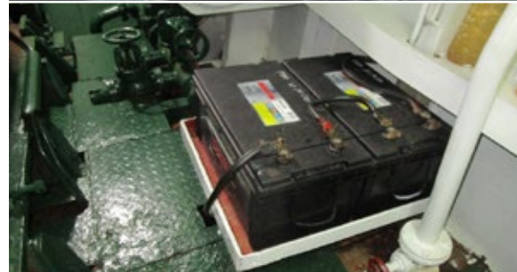
! Poor installation of batteries.
