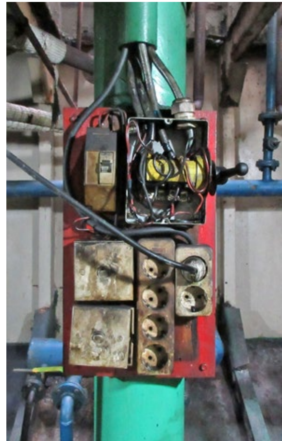
! Live components should not be exposed.
