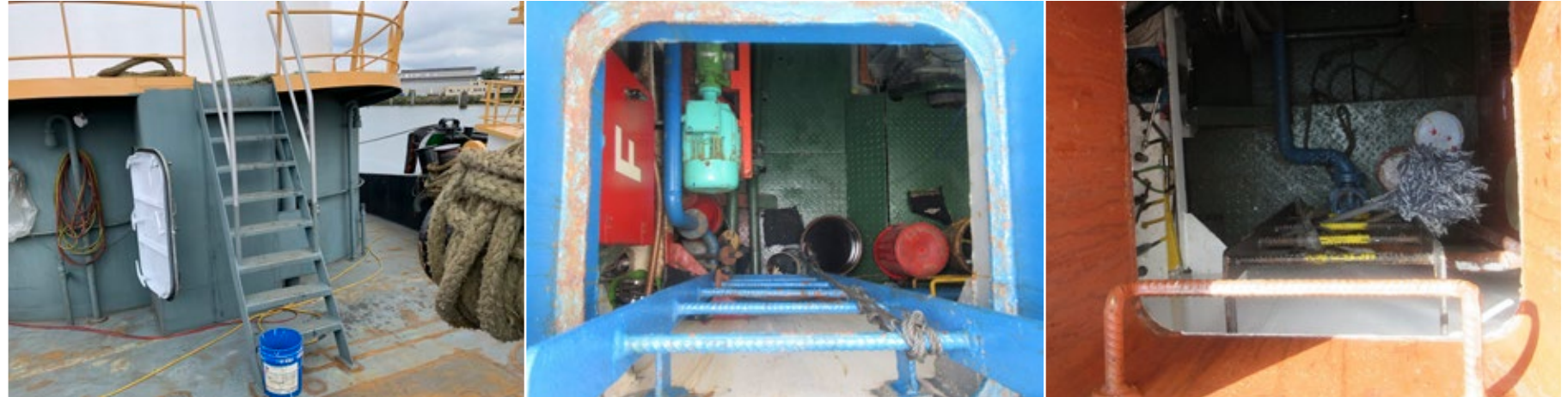
! Trip hazards at the top and bottom of ladders.
