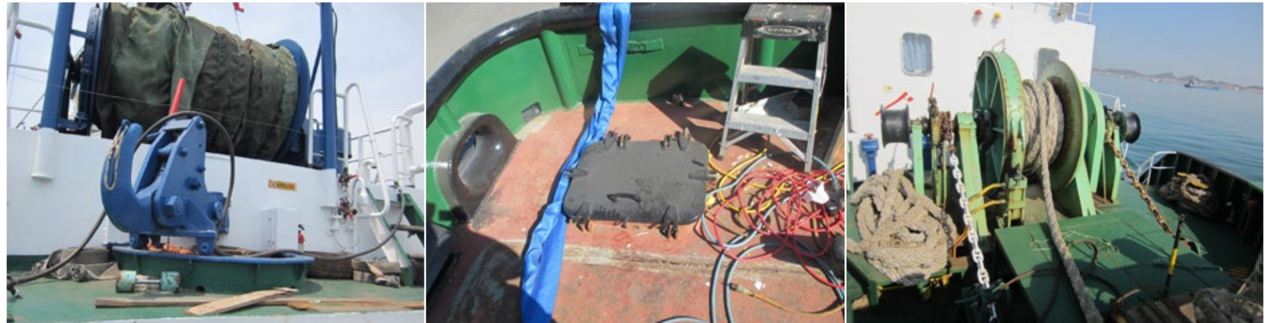
! Trip hazards on deck.
