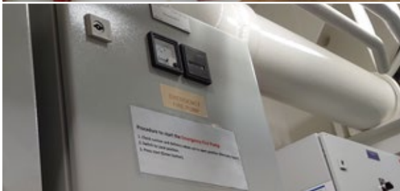
Control panels and valves in good condition, clearly signed and labelled, and operating instructions posted.
