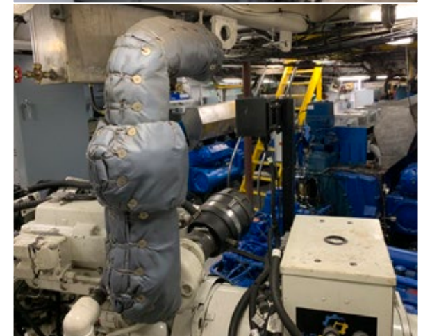
! Insulation in good oil-free condition and tightly fitting with no gaps exposing hot surfaces.
