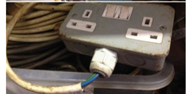
! Cable terminations should be secure. The cable jacket should be secured inside the termination – individual wires/conductors should not be exposed and junction boxes should not be taped in place.
