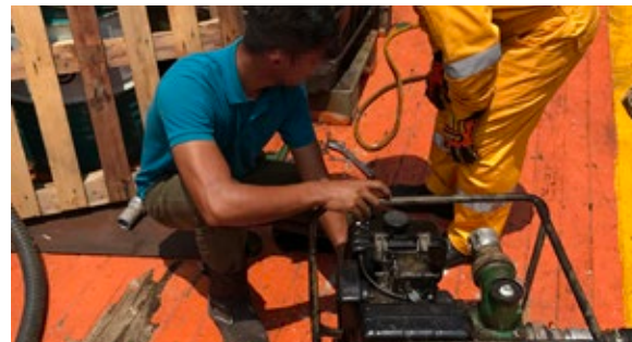
! Crew spent more than 20 minutes trying to get this emergency generator started and never succeeded.
