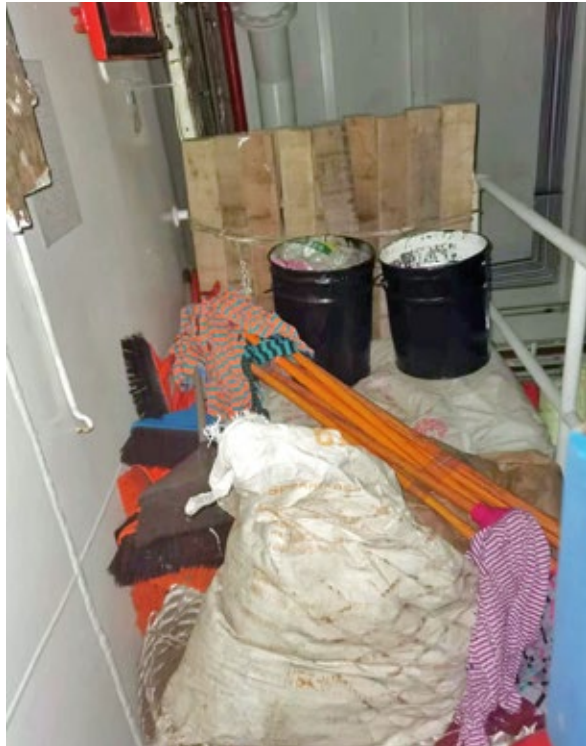
! Clutter making unsafe access to the vent flap.
