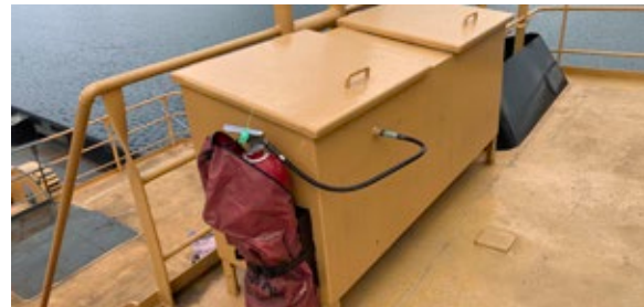
Portable and wheeled (mobile) fire extinguishers exposed to weather are protected, and are subject to routine inspection and periodic renewal.
