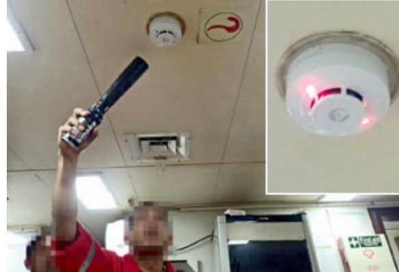
Fire detection and alarm system regularly tested, by appropriate means.
