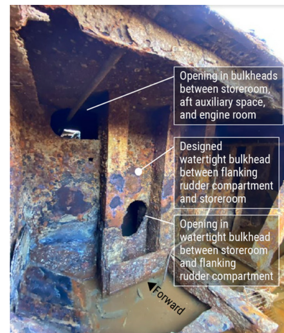
Figure 112. Flanking rudder compartment after recovery. Openings in bulkhead shown are also typical of other bulkheads below the main deck separating compartments. BACKGROUND SOURCE: COAST GUARD
