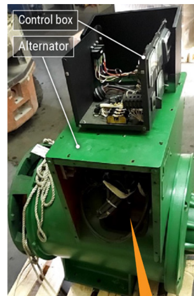
Figure 125. Below: Close-up of port alternator terminal block showing damaged connection and metal arcing residue accumulated on terminal block posts. Detail shows the severed wiring harness.
