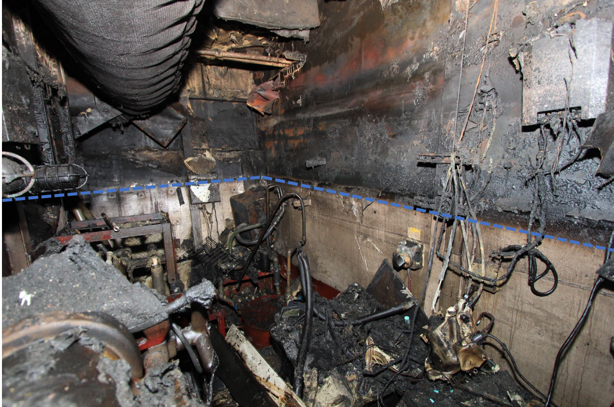
Figure 9. Portside engine room bulkhead exhibiting demarcation line ( dashed blue ) between thermally damaged and undamaged area.
