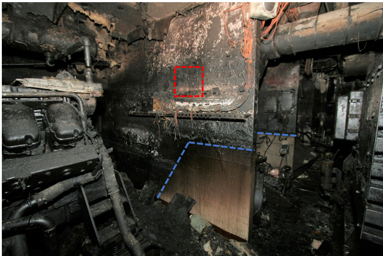
Figure 10. Bulkhead forward of port main engine with low-lying damage towards the outboard side. Demarcation line ( dashed blue ) and original location of electronic throttle controller ( red ) shown.
