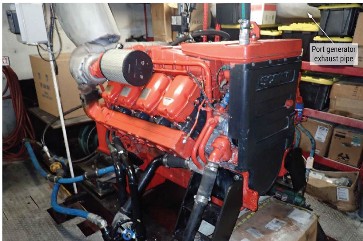
Figure 11. Photo from survey on June 2, 2022, showing port main engine ( foreground ) and storage shelf. The white port generator exhaust pipe is visible behind some of the boxes on the shelves. (Source: Knox Marine Surveyors & Consultants)
