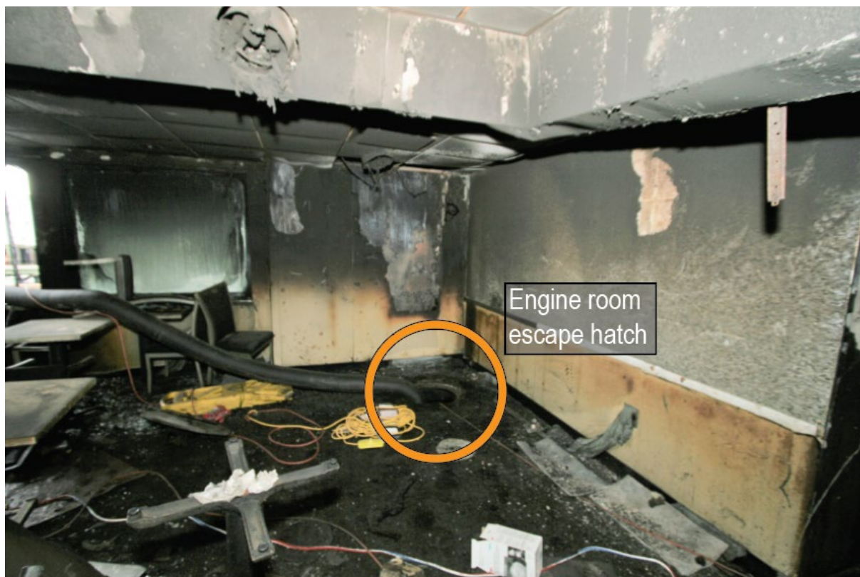
Figure 15. Photo of the engine room escape hatch on the main deck after the fire.
