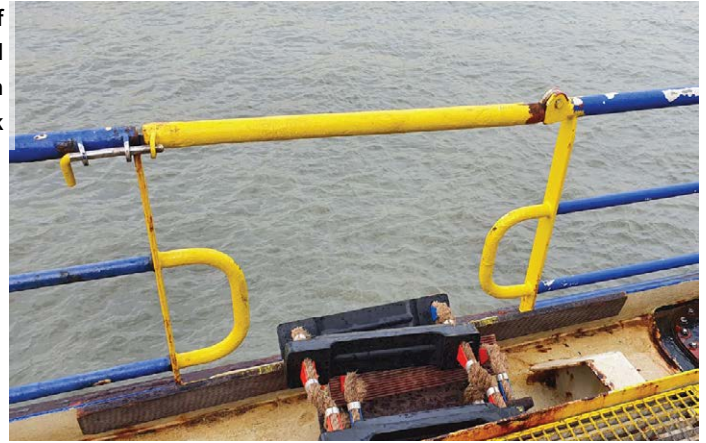
Figure 4: Second example of a noncompliant handhold stanchions for the transition from pilot ladder to deck
