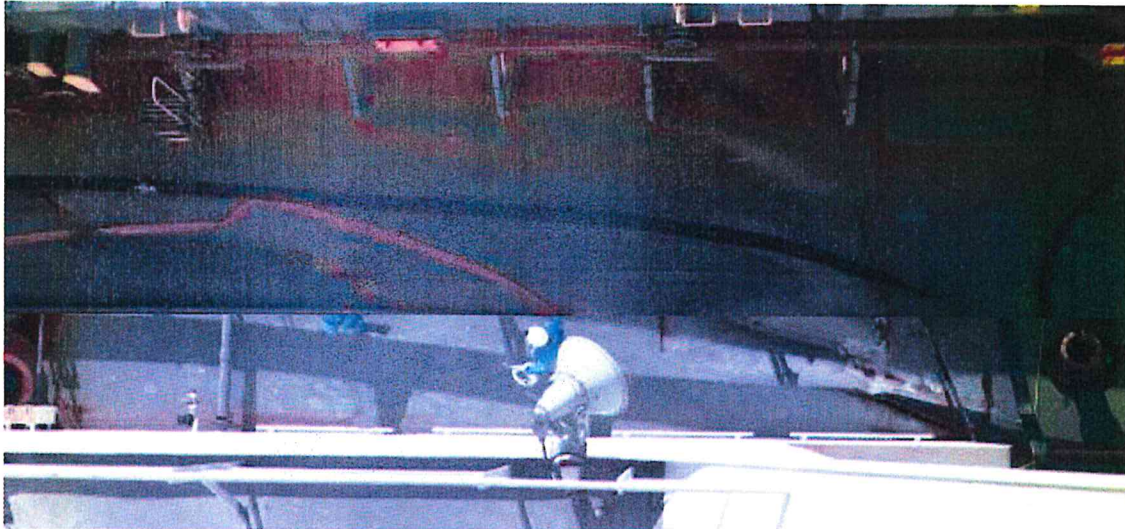
Figure 14, SB crack at frame 42-46 on main deck.
