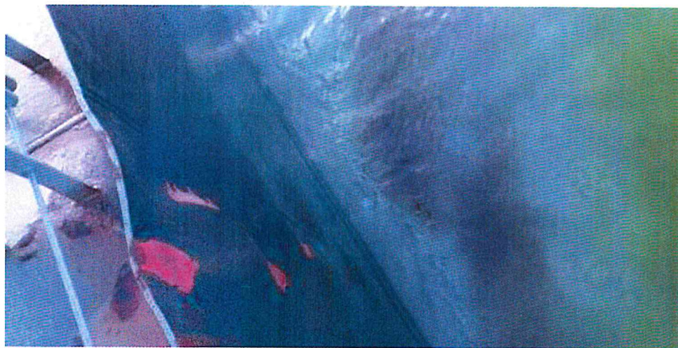
Figure 10, SB buckling at frame 60, view from deck
