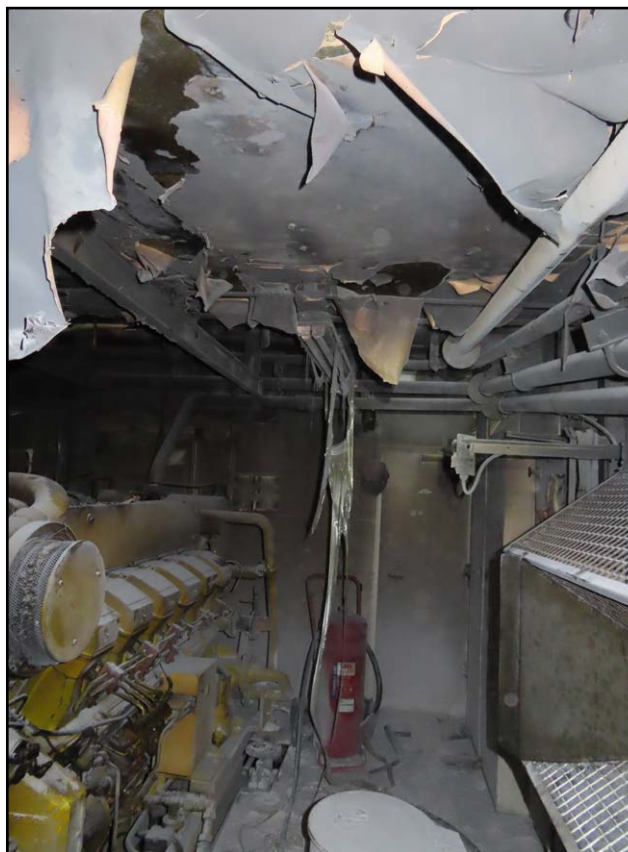
Finnmaster's fire-damaged compartment
