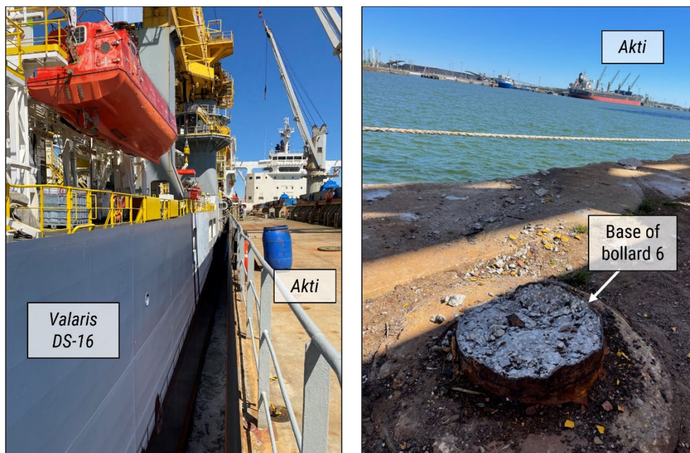
Figure 7. Postcasualty photos showing VALARIS DS-16 alongside the Akti after making contact ( left ) and the remaining base of bollard 6 after breakaway ( right ). (Source: Coast Guard)
