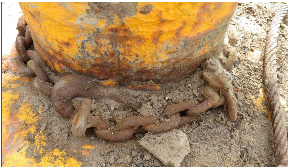
Figure 10. Steel chain wrapped around base of bollard 7 after the casualty. (Source: Coast Guard)
