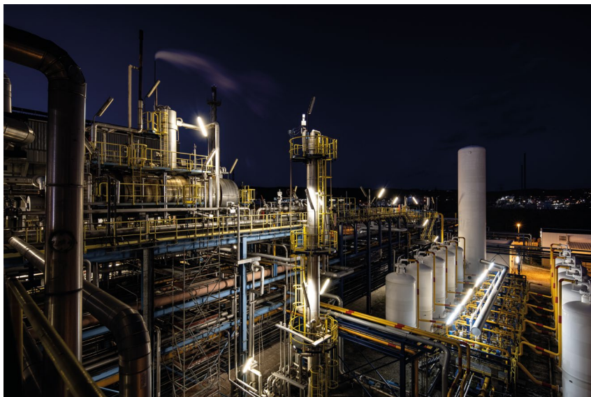
Steam methane reforming hydrogen production site in Port-Jérôme (Source: Air Liquide)
