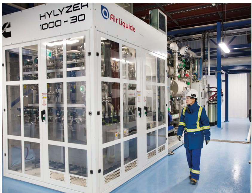
HyLYZER - electrolyser system (Source: Air Liquide)
