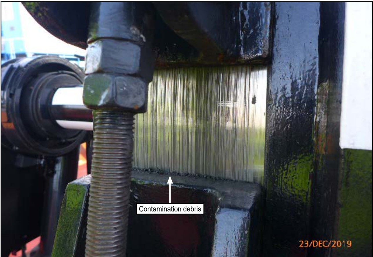
Figure 18: Starboard forward winch brake contamination
