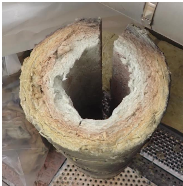
Figure 18 Cross-section of fire-affected thermal insulation on the overlying PL-13-0718 pipe. Source: Equinor
