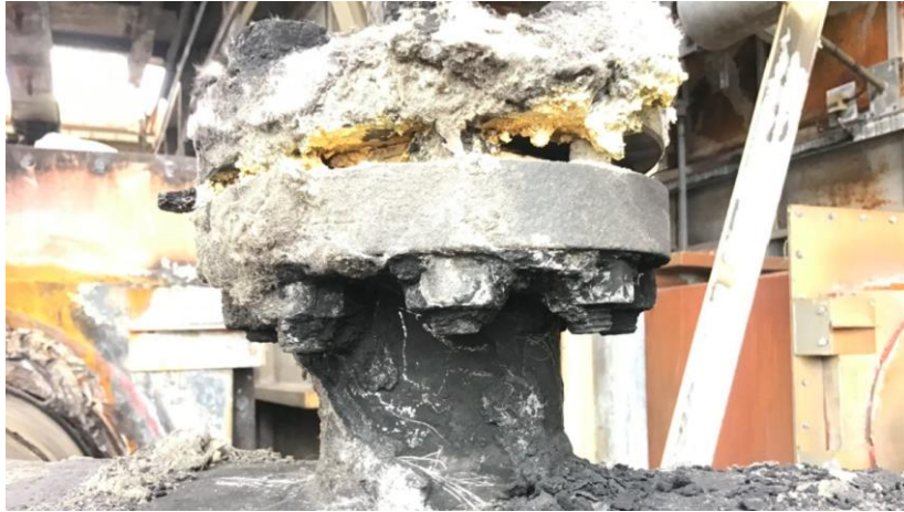
Figure 13 The two-inch thermowell flange after the fire. Source: PSA
