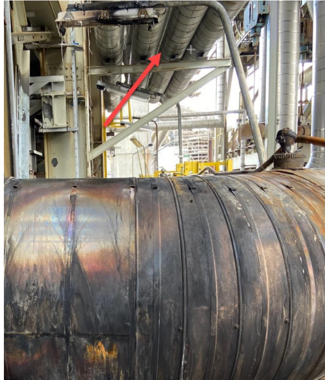
Figure 17 PG-14-0204 and overlying pipe tracks immediately above the leak point. Source: Equinor
