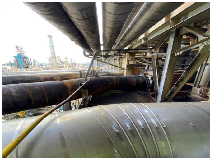
Figure 12 The fire area, with the thermowell where it started in the centre. Source: Equinor.
