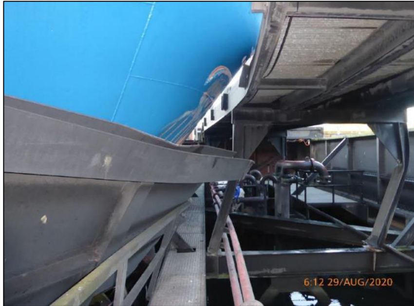
Figure 7: Damage to the lock gate (close-up 1) 23
