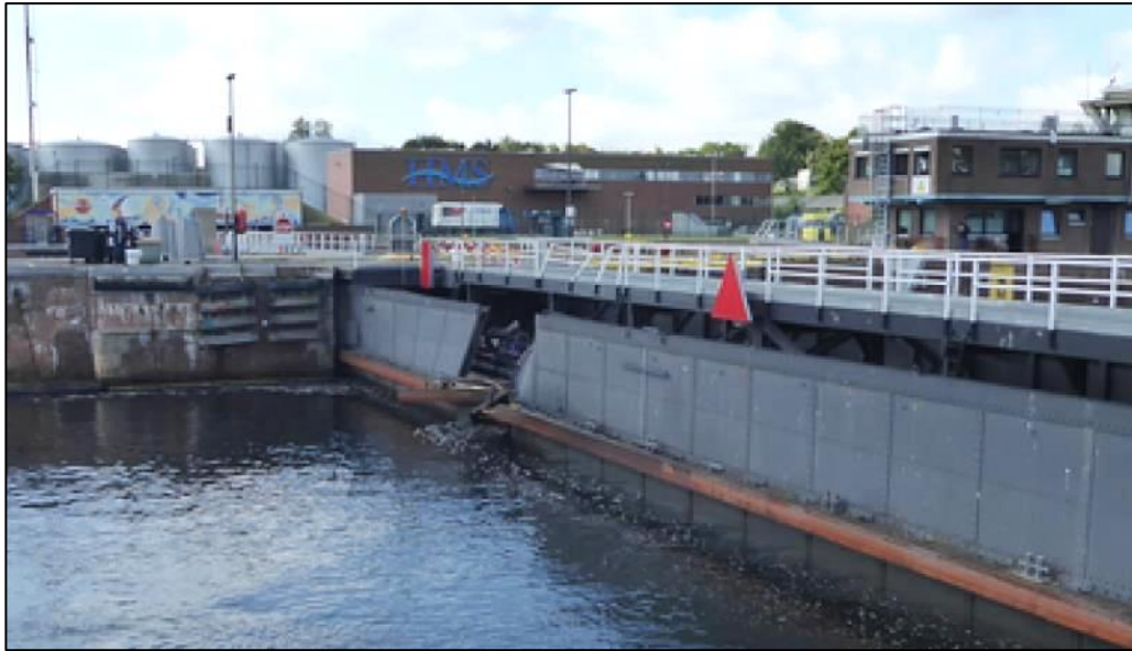
Figure 9: Damage to the lock gate (general view) 24
