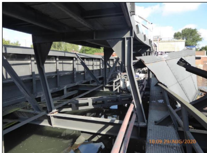
Figure 8: Damage to the lock gate (close-up 2)
