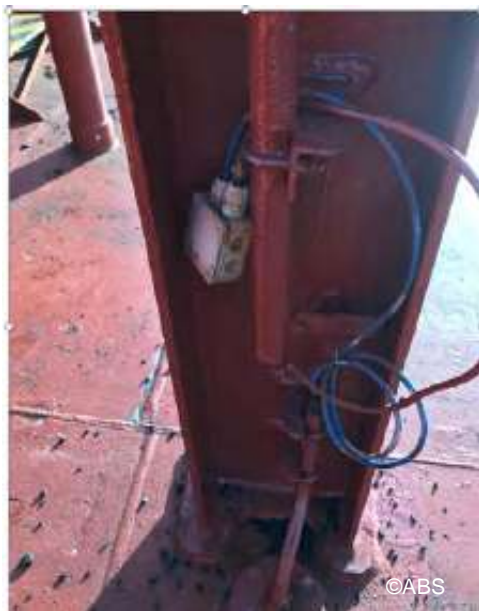
Electrical connection box not secured
