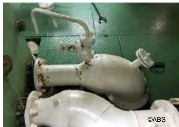
Main Fresh Water cooler inlet pipe leaking
