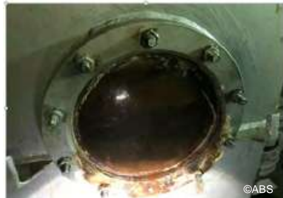
HT Water expansion tank sight glass leaking
