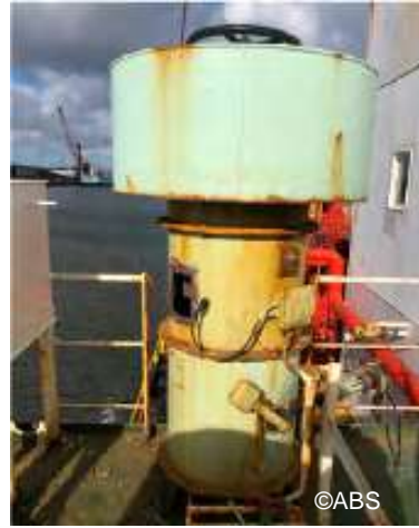
ER ventilation fan damper unable to operate
