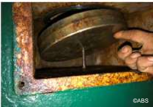
Tank vent disk wasted
