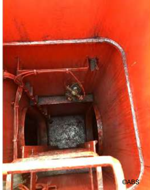
Loose/broken lighting inside vertical trunk
