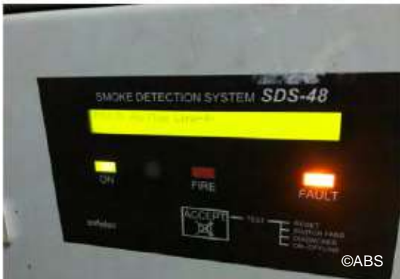
Cargo Hold Smoke extraction system faulty
