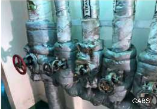
Handwheel missing, lagging damage
