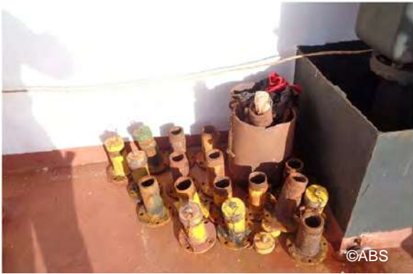
Sounding pipe for cargo hold bilges (several) thread wasted
