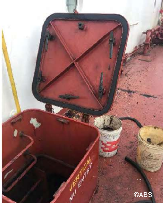
Missing Dog for watertight hatch cover
