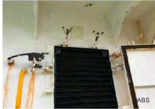
Watertight indication sensor not operational
