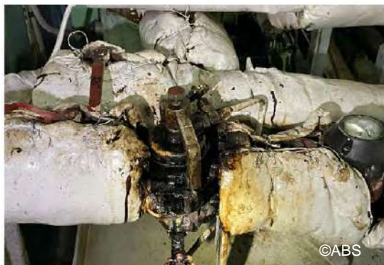
General condition of ER, with oil in transfer pump filter
