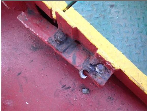
Figure 10: One nut had been successfully cut by the angle grinder, before the explosion occurred
