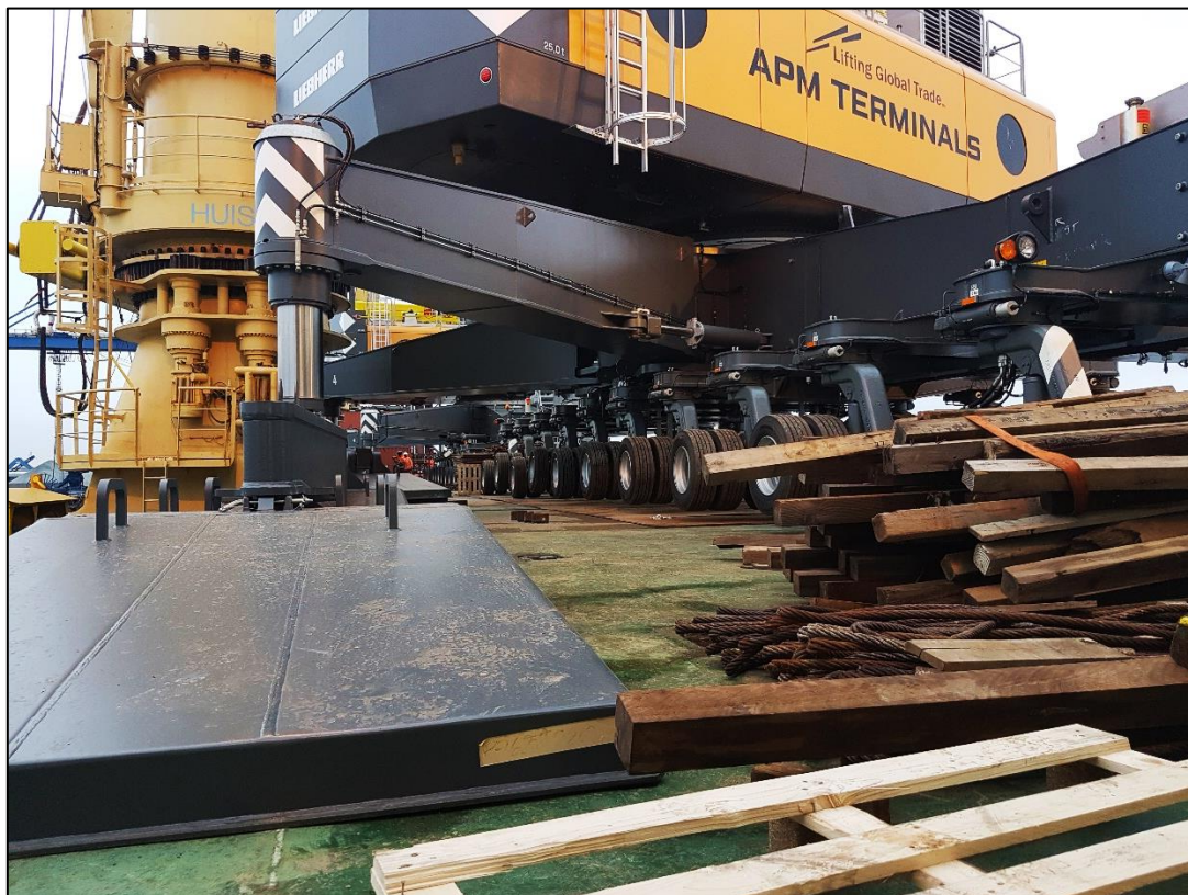
Figure 8: View from the deck looking towards the stern after the two cranes were loaded
