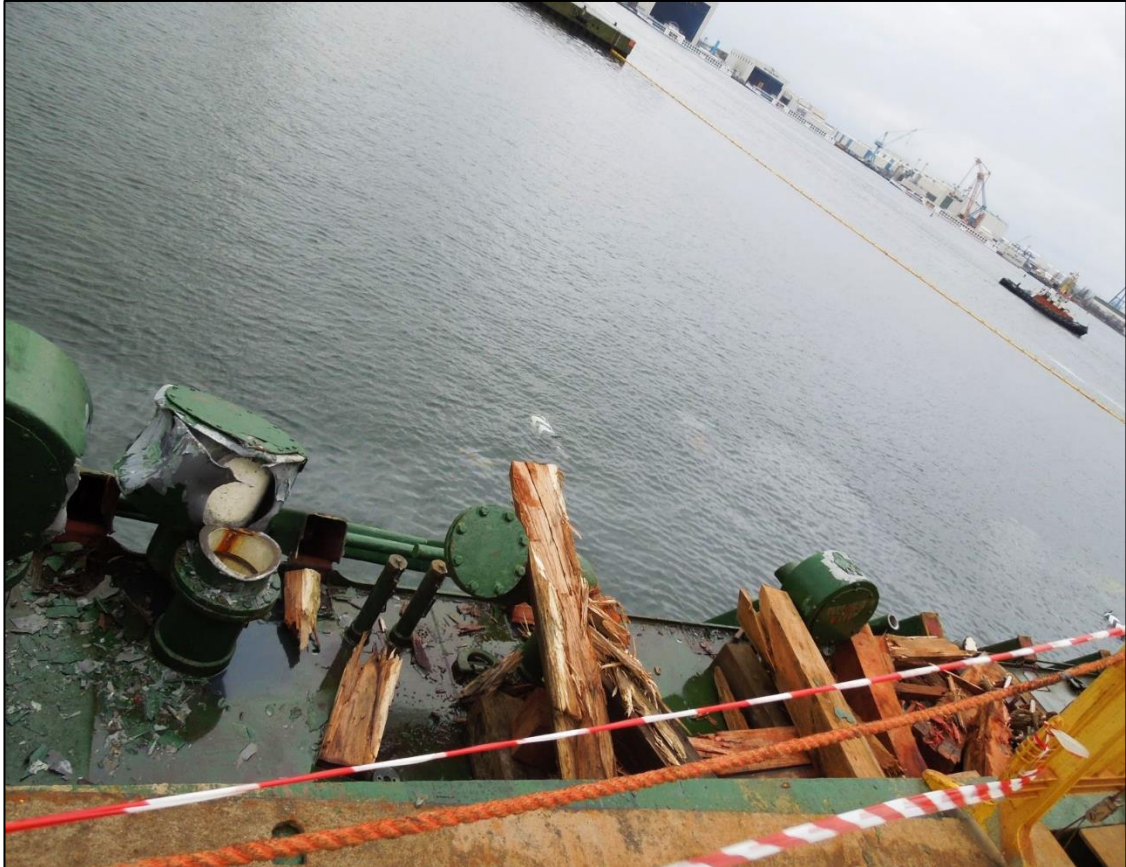
Figure 13: Damage to port-side deck passageway caused by crane 2 (sounding pipes, vent heads, overflows, wooden blocks, missing railing)
