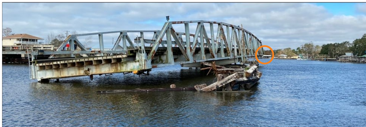
Figure 7. Postaccident damage to Barataria Bridge looking north. The corner of the swing span that the barge contacted is circled. (Source: anonymous)
