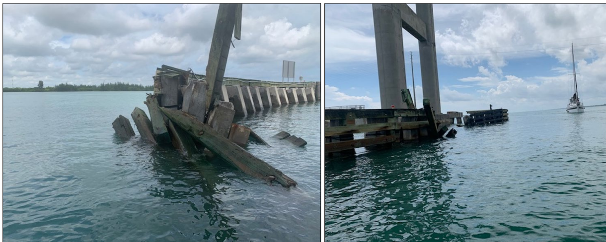
Left: Postaccident damage to the eastern fendering of the bridge looking to the north. Right: Postaccident damage to the eastern fendering of the bridge looking to the south. (Source: Coast Guard)
