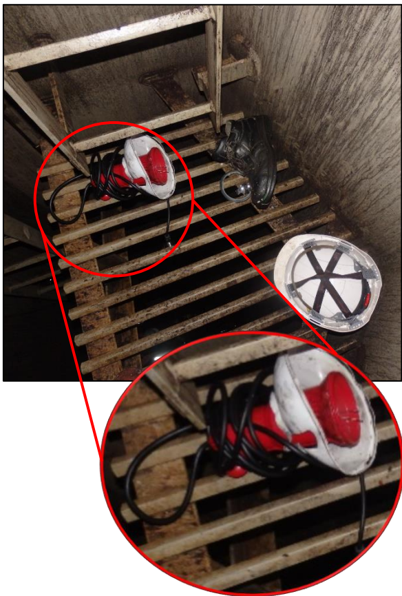
Figure 5: Portable light, safety shoe and safety helmet as found on platform C
