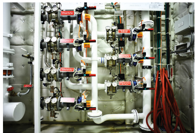
Figure 10: Water spray system valves for vehicle deck
