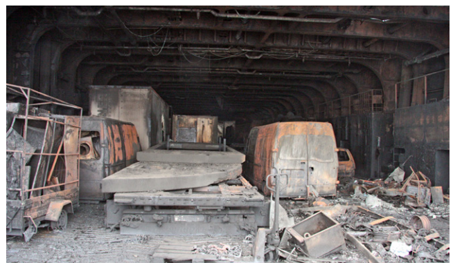
Figure 23: Garage space fire © Central Command for Maritime Emergencies, Germany
