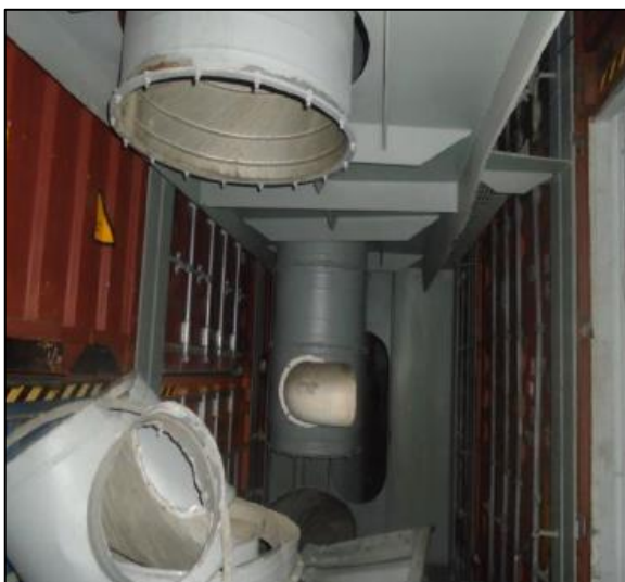
Figure 4: Mechanical ventilation duct damaged
