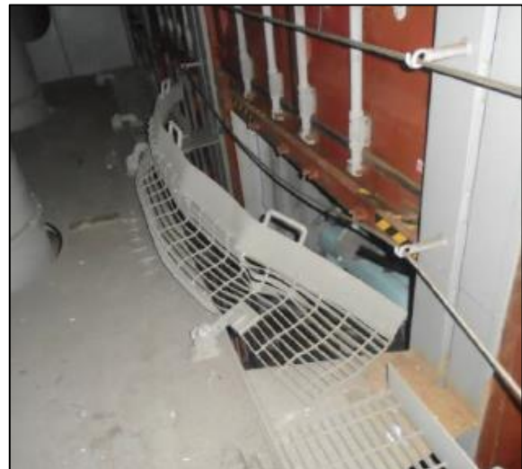
Figure 5: Distortion of steel walkway platform
