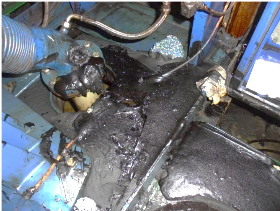
Figure 4 - Sludge gushed out of the inspection opening
