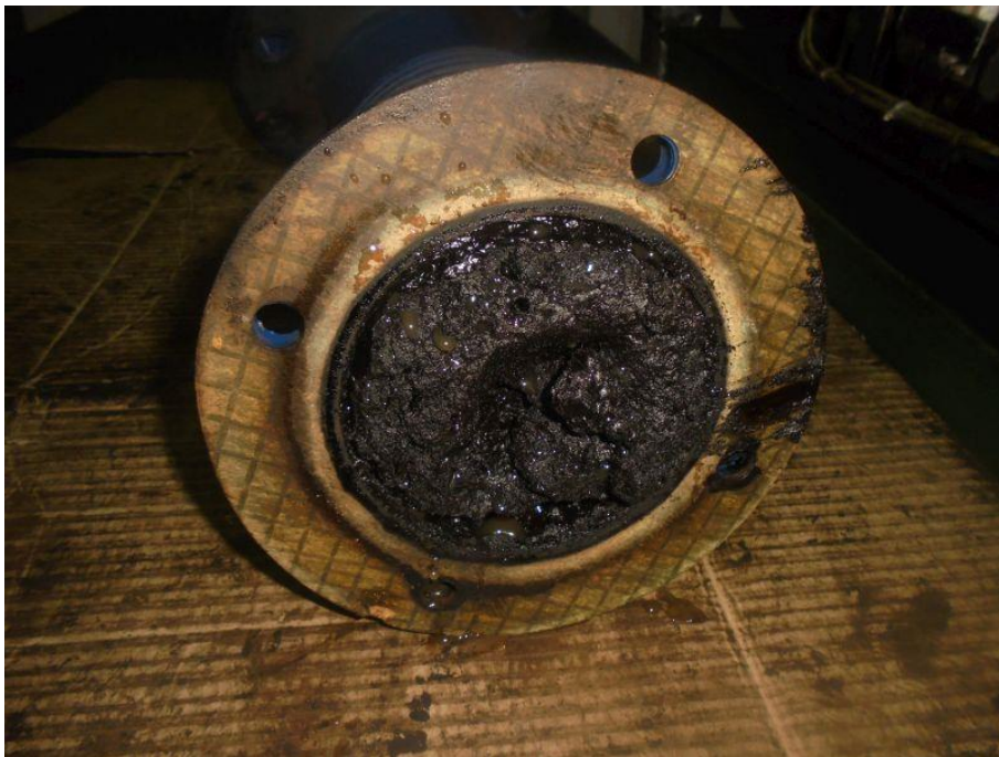
Figure 7 - Completely blocked sludge discharge line of separator N°1
