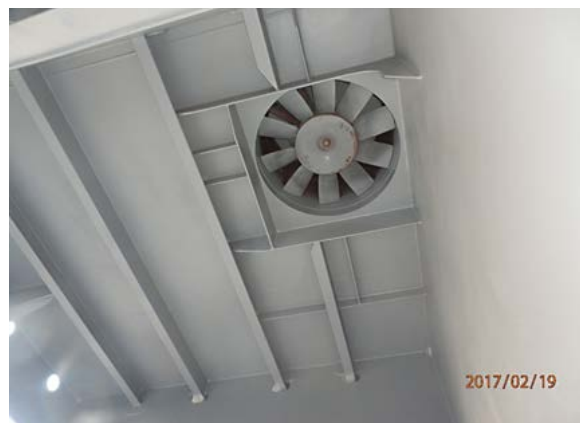
Figure 8: View of cargo hold mechanical ventilation impeller from inside the cargo hold - cross-deck (photo courtesy of Ionic Shipping (Mgt) Inc.)
