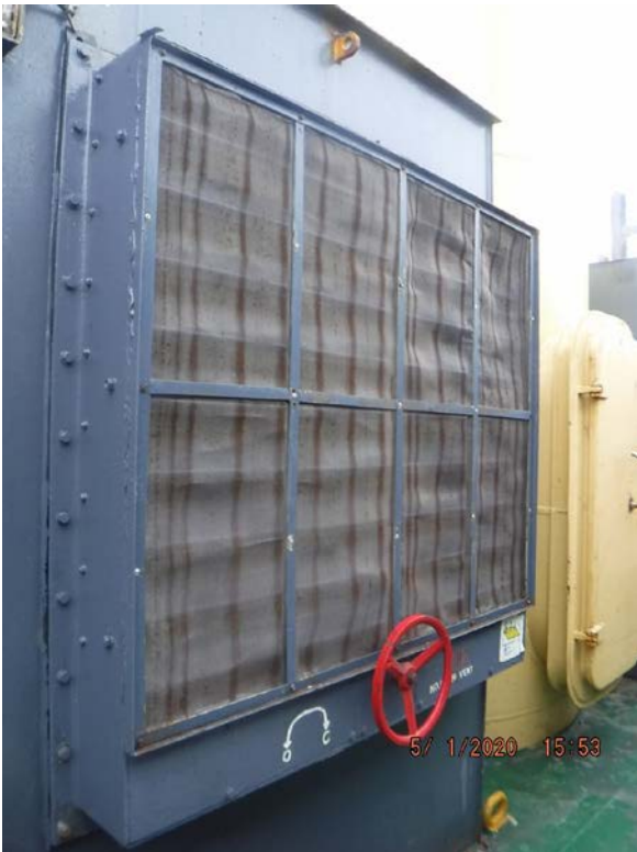
Figure 12: Mechanical ventilation with integrated closing damper (photo courtesy of OLDENDORFF CARRIERS GmbH & Co. KG.)
