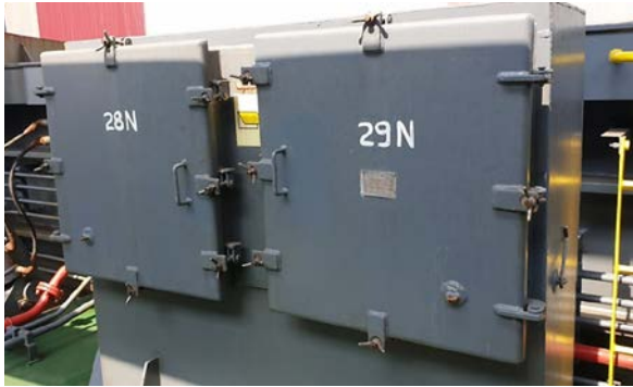
Figure 3: Hinged-door natural ventilator in casing on main deck (photo courtesy of OLDENDORFF CARRIERS GmbH & Co. KG.)
