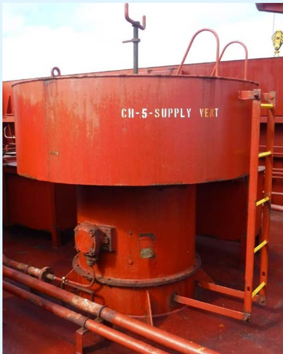
Figure 9: Mechanical mushroom-type ventilator (photo courtesy of Liberty Maritime Corporation)
