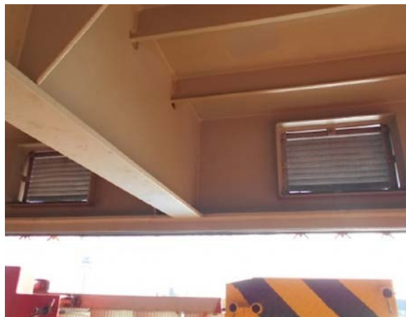
Figure 2: Internal view of hinged-door ventilator on cargo hold hatch cover side (photo courtesy of Optimum Marine Management Ltd.)
