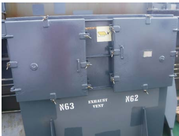
Figure 6: Hinged-door mechanical ventilation - exhaust vent (photo courtesy of OLDENDORFF CARRIERS GmbH & Co. KG.)
