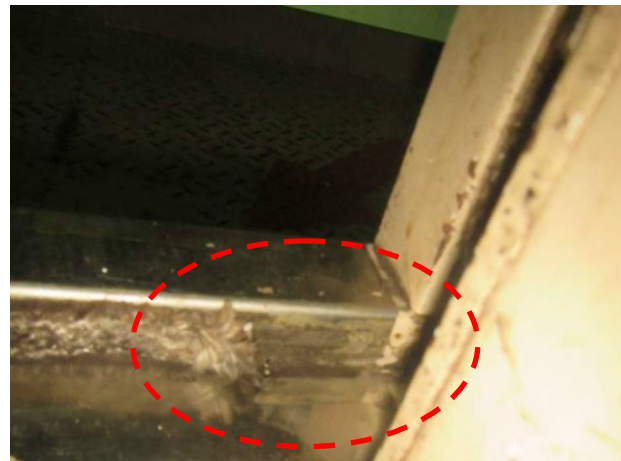
Missing fire door packing →
