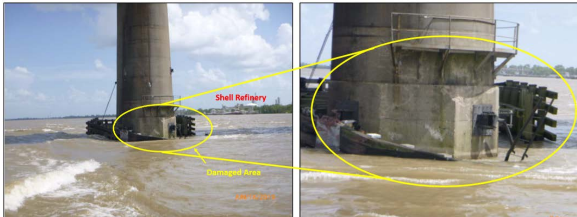
Damage to the fendering system for the western pier of the Sunshine Bridge, from the north. (Source: Louisiana Department of Transportation and Development)
