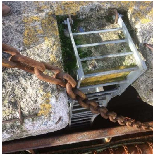
Figure 10 - Chains of fishing gear obstructing quay side ladder (2)
