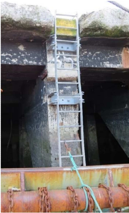
Figure 4 – Quay side ladder at the berth of fv Z.15 - ZILVERMEEUW
