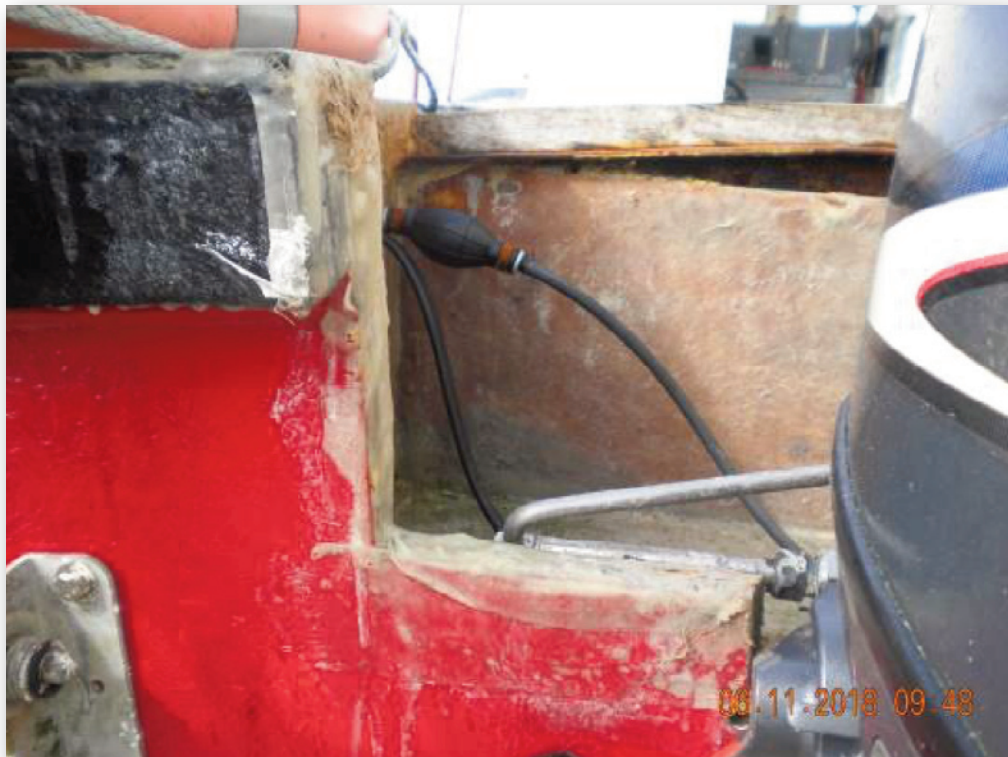
Photograph No. 5: Cut out section of transom with fibreglass used to seal joint.
