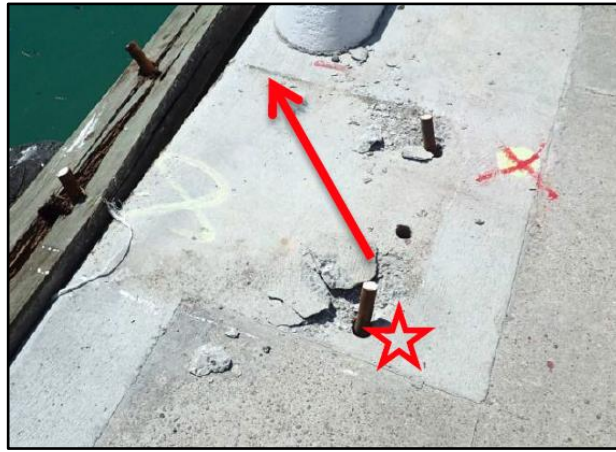
Figure 9 Bollard 26 after the failure, showing the direction of mooring lines to the ship
