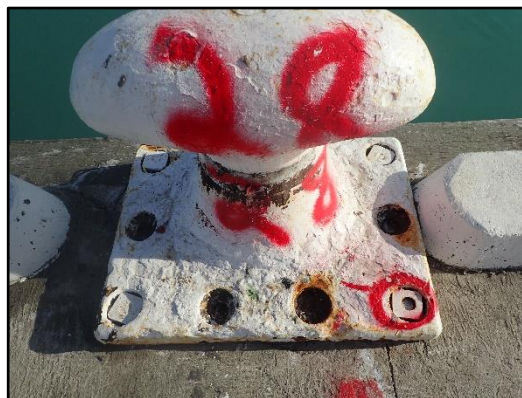
Figure 12 Underutilisation of the bollard securing arrangement
