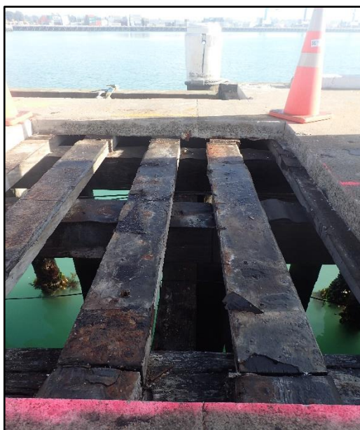
Figure 7 Number One Wharf – ‘hit and miss’ decking under concrete
