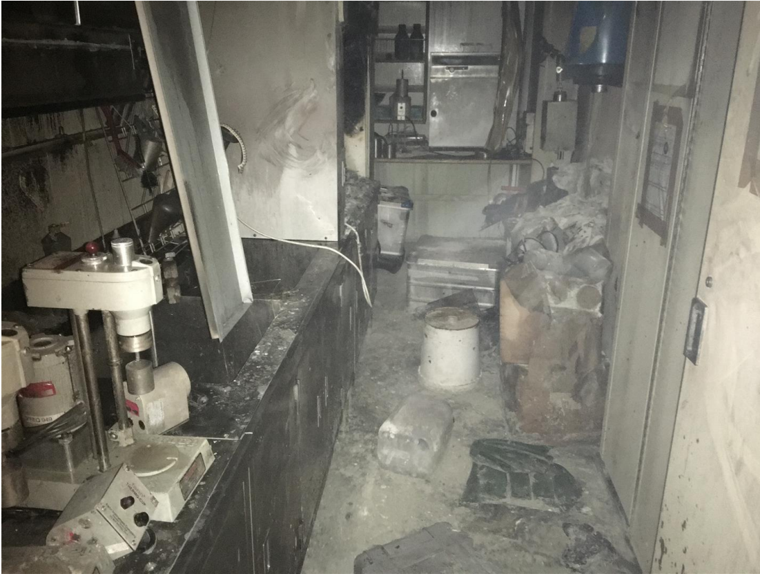
Figure 4 Overview of the mud lab after the fire (from Seadrill).
