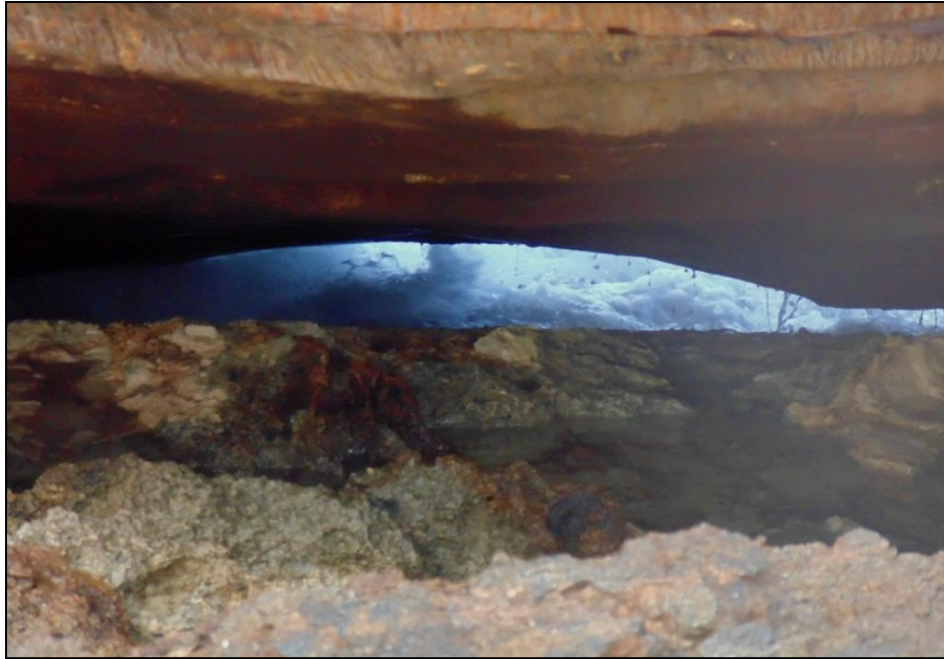
Figure 9: Bottom shell plating damage
