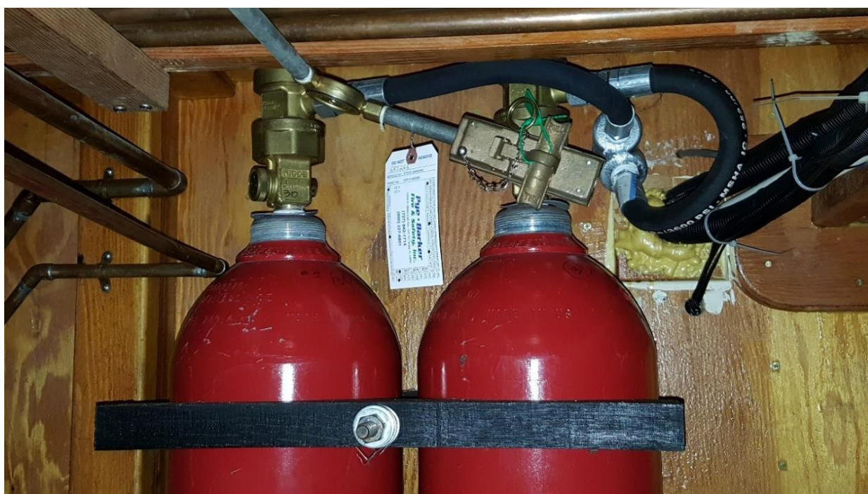
Figure 18. Components of the Island Lady 's fixed fire suppression system in March 2017 before the fire. (Photo by the Coast Guard)
